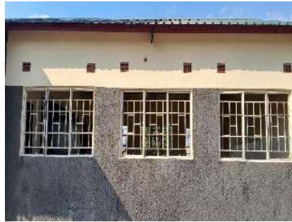
Windowpanes not fitted
