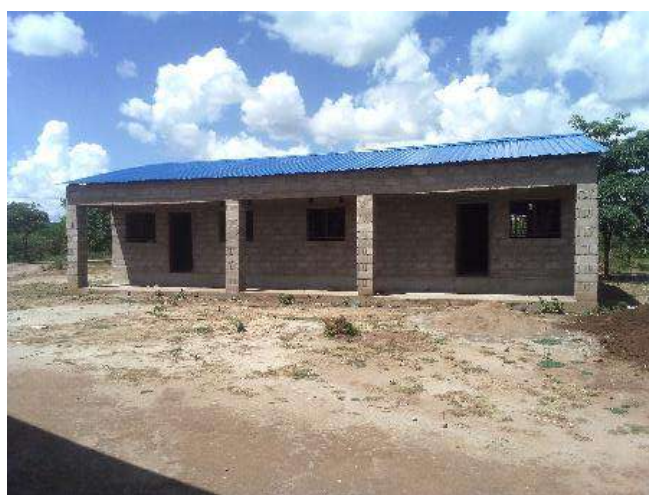
Incomplete and abandoned Maternity ward at Magobo
