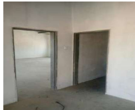
doors not fitted on the classroom and Office
