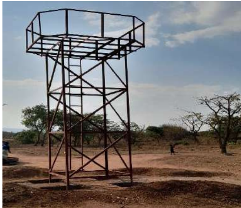
Incomplete water reticulation
