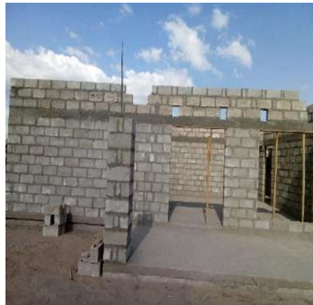
Incomplete Chinsanka Police Post
