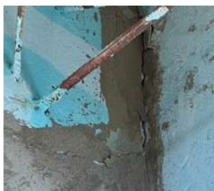
Crack on Concrete Pad
