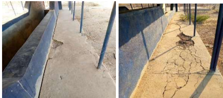
Poor workmanship – Construction of dip tank.
