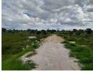
Incomplete works at Moboshi bridge
