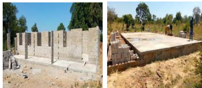
Dormitory at ring beam and dormitory at slab level – Nyawa Secondary School
