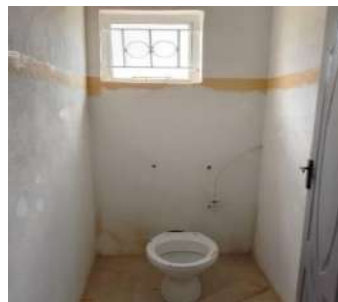
Toilet without cisterns
