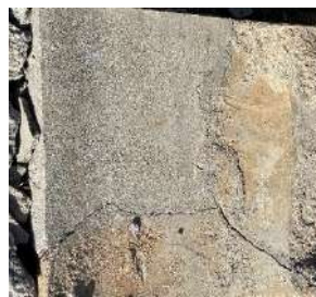
Crack on Spoon Drain
