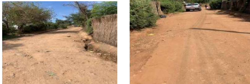
Washed way side drains and spot gravel
