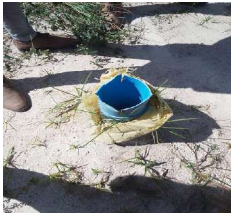
Vandalised casings at Mukalizi Primary School
