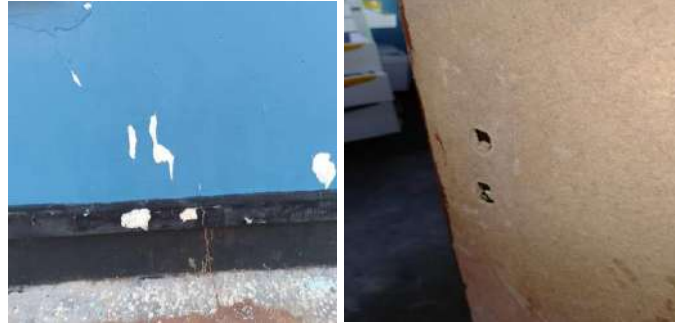
Paint Peeling off
