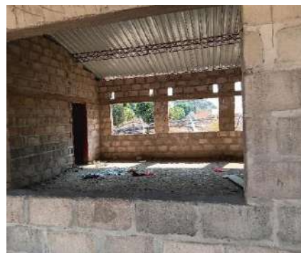
Windows and air vent not fitted
