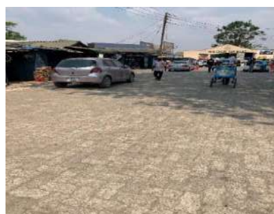
worn out pavers
