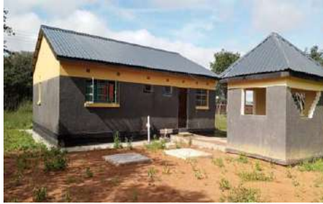
Staff House without power connection
