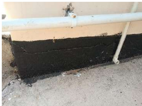
Cracks in the foundation box
