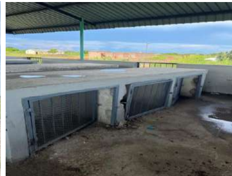
Vandalised Grill gates
