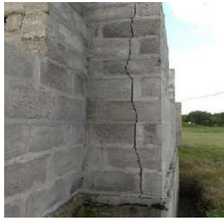
Cracked wall 1x3 CRB
