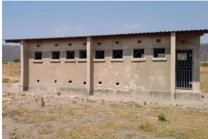
Incomplete Ablution Block
