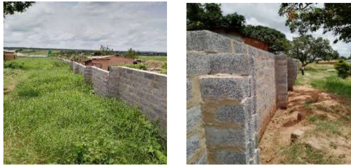
Incomplete wall fence
