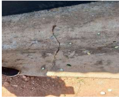
Cracks on the Spoon drainage
