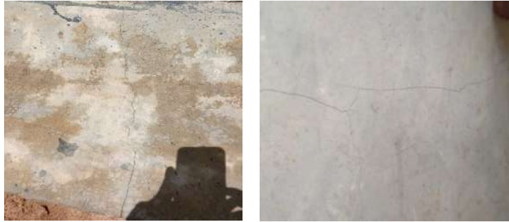
Cracks on the Spoon Drain and Floor
