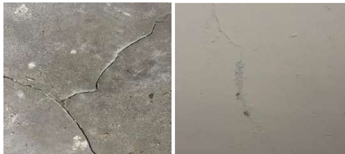
Cracked floor and wall at the staff house and classroom block
