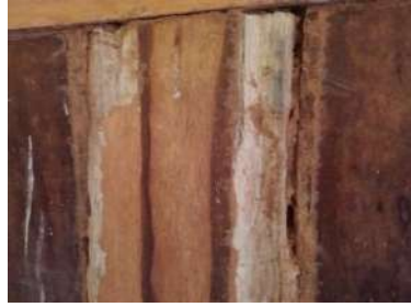
Door Exposed to Termites
