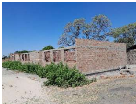
Side view of the CRB
