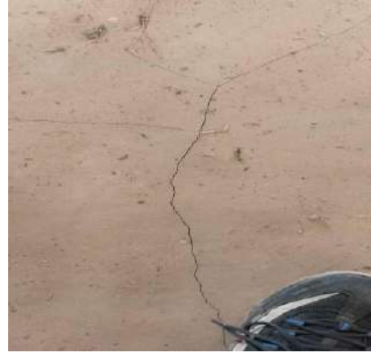
Cracked Floor in the Classroom
