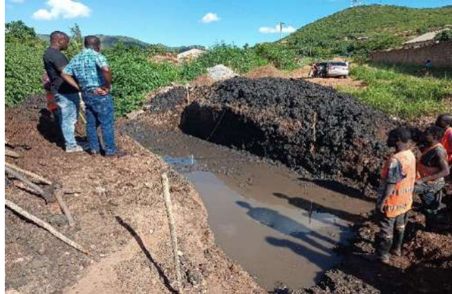
Delayed Completion of the Chizongwe Foot Bridge
