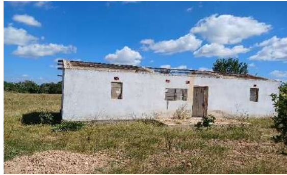
Blown off roof at Singani East Primary School
