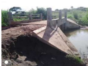
Eroded part of the bridge
