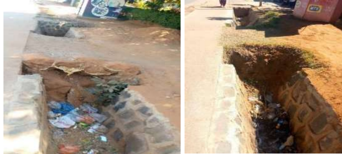
Crossing Points into Residents not done
