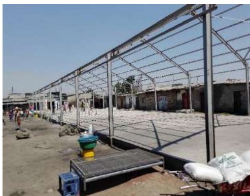
Incomplete Traders Shelter
