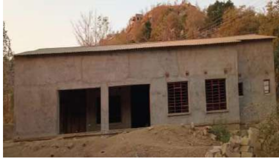
Incomplete Kaleya Clinic
