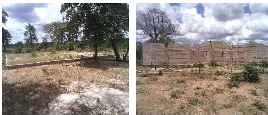
Incomplete works at Mtsanya Health post
