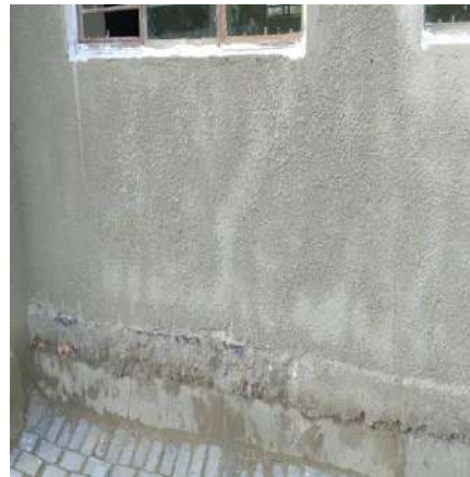
Peeling off plaster
