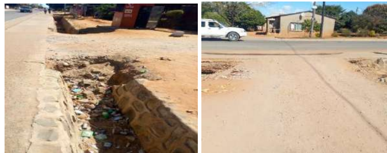
Crossing Points into Streets not done
