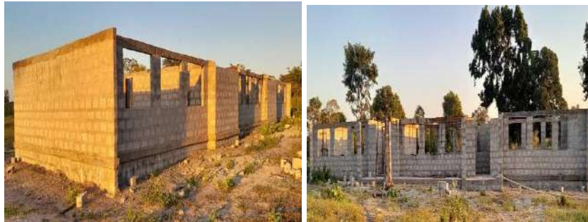
Incomplete and stalled works
