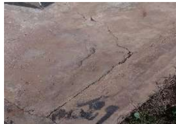
Cracked Spoon Drain
