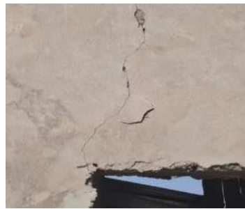
Cracked Plastered Wall
