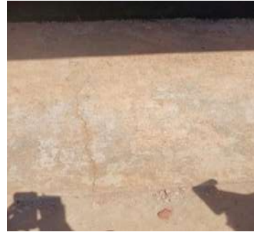
Cracks on Veranda
