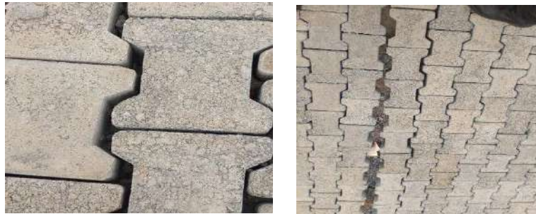
Failure to Lock Pavers
