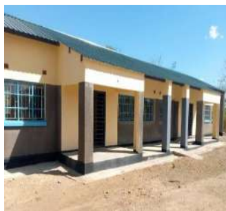
1 x 3 classroom block not handed over
