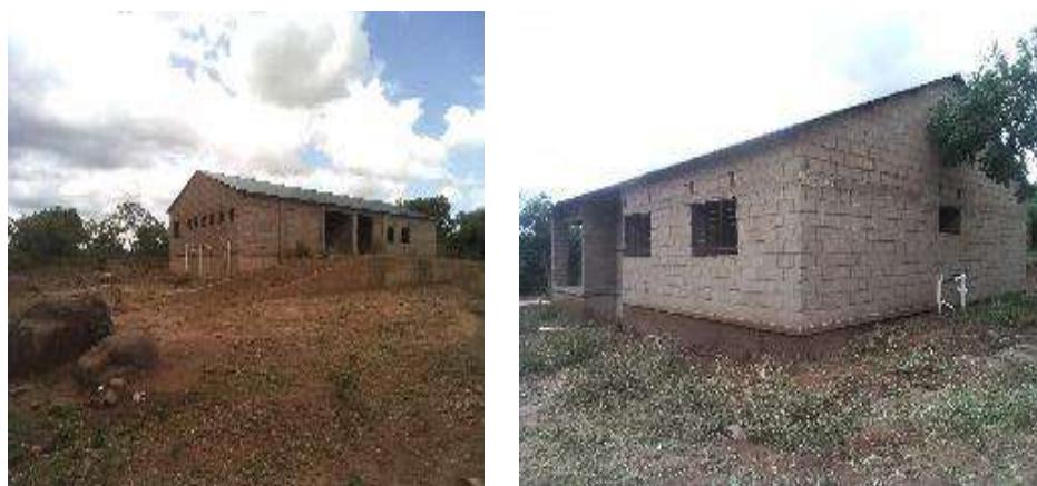
Incomplete Works at Mkale Health post and House
