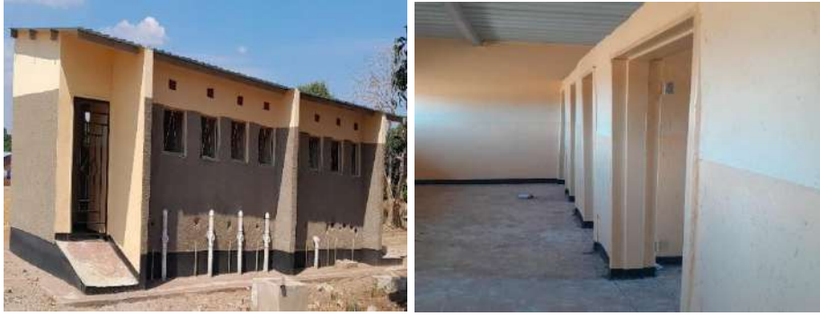
Incomplete ablution block
