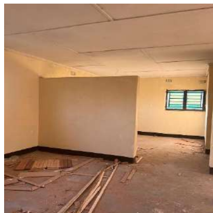
Installation of Bunker Beds not done
