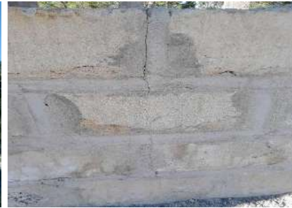
Cracked wall of 1x3 CRB
