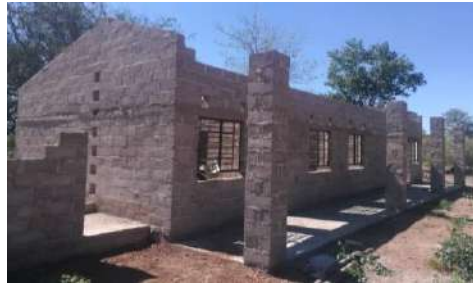
Delayed completion – Lunungu Maternity Annex
