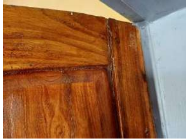
Hard wood door with cracks
