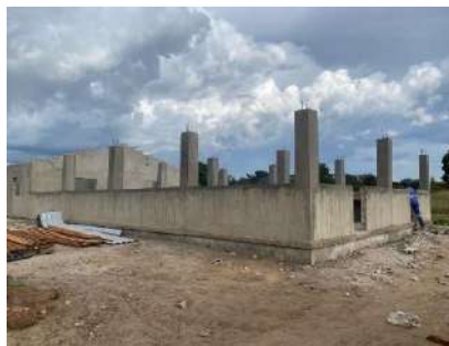
Uncompleted Market Shelter at Kalamba
