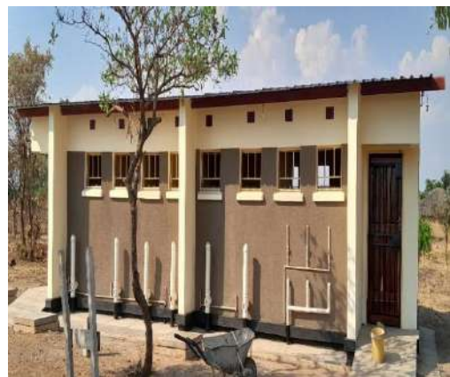
windowpanes not fitted
