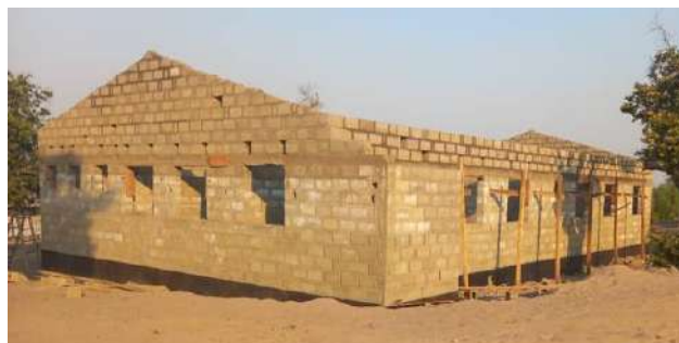
Incomplete Maternity Wing
