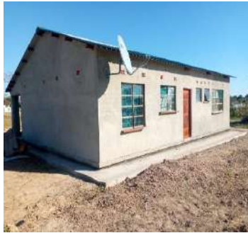
Air vents and glass Panes not fitted
