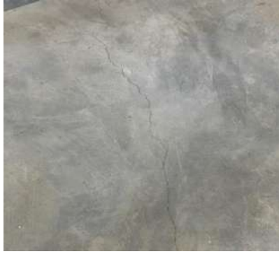
Cracks on the Floor
