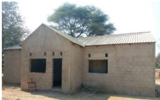
Stalled Project – Maamba Police Cells
