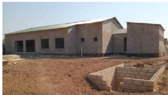
Incomplete Chalokwa Rural Health Post
