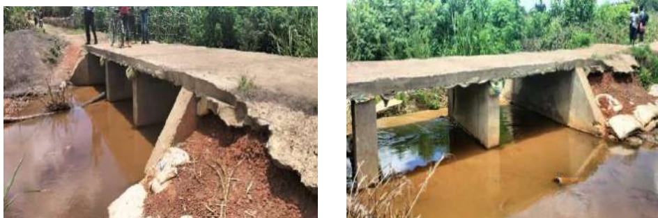
Incomplete Bridge at Mishishi Stream
