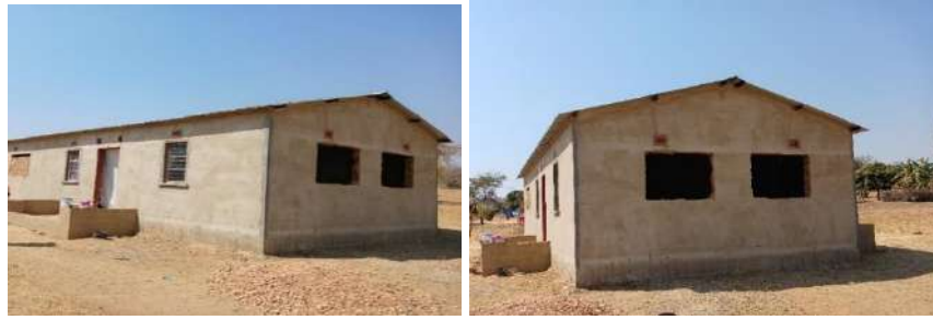
Incomplete Staff House at Siasikabole Primary School
