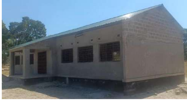
Incomplete Construction of 1x2 CRB at Mulonga Primary School
