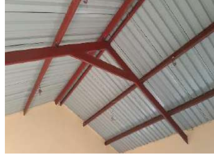
Electrical installations not installed
