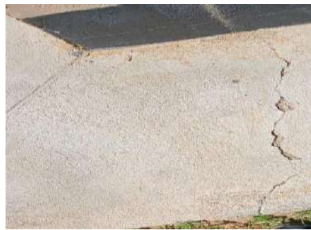
Cracks on the Apron
