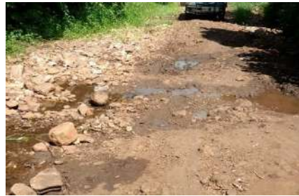
Water ponding at 1.6Km
