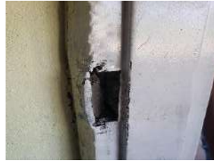
Poorly fabricated door frame
