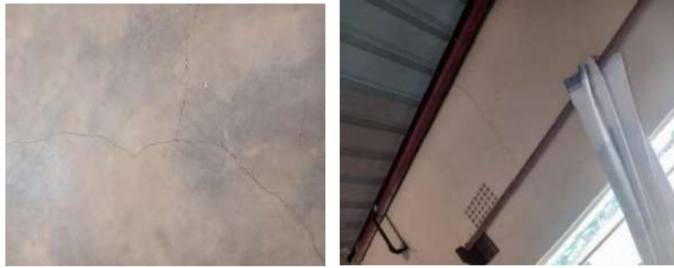
Cracks on the Wall and Floor
