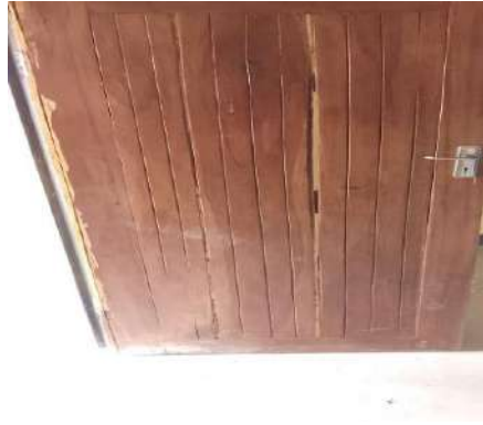
Cracked Soft Wood Door
