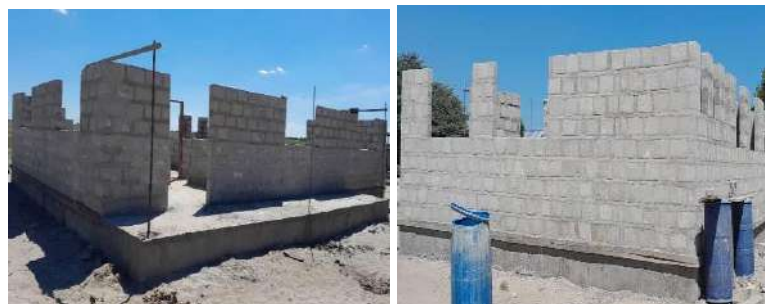
Incomplete maternity wing
