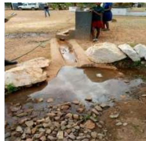
Soak Pit Overflowing at Mutamba Primary School
