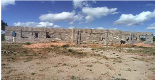
Incomplete Police Post at Kagoro
