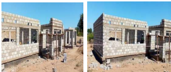
Incomplete 1 x 3 classroom block
