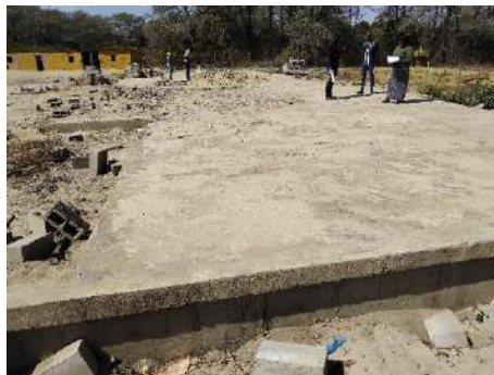
An abandoned slab eroding at the centre
