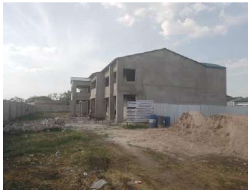
Twashuka Combined School Incomplete Structure
