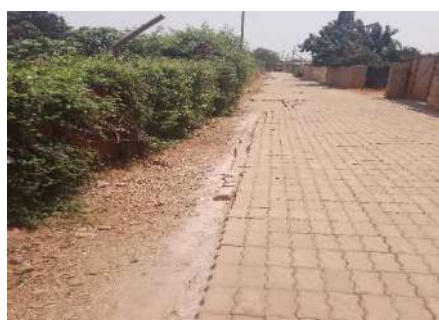
Incomplete Christon Tembo Road
