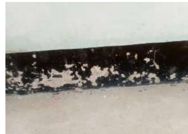
Paint peeling off
