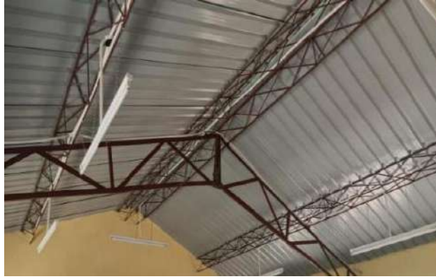
1x2 CRB roof without ceiling board
