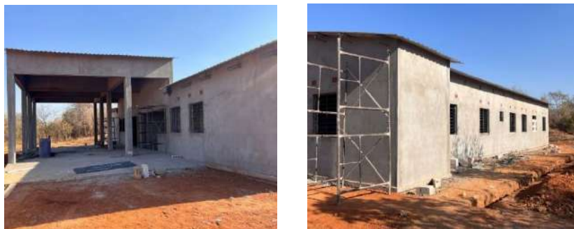
Incomplete Rural Health Post
