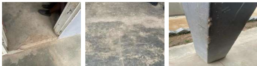
Floor cracks and poorly plastered pillar
