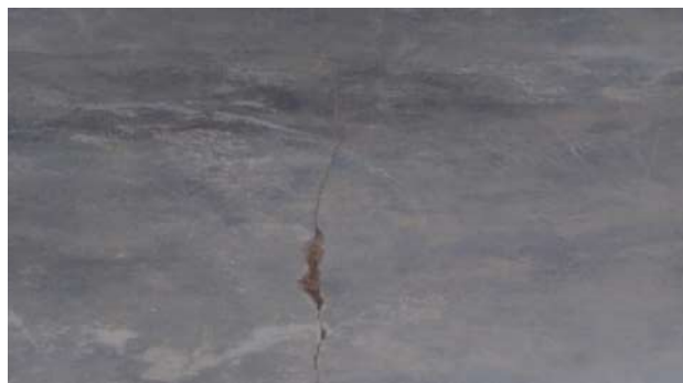
Crack on the Front Apron of the 1 x 3 Classroom Block
