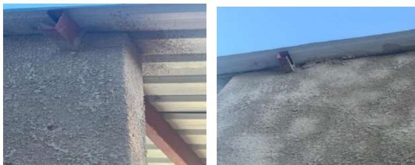
Improper Fitting of Trusses Causing Cracks in the Wall
