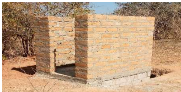
Incomplete VIP Toilet
