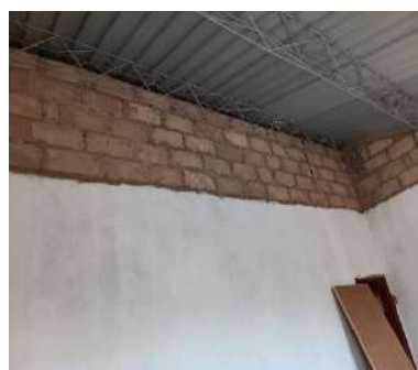
Incomplete plastering works
