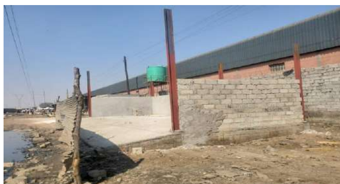
Incomplete Garbage Bay
