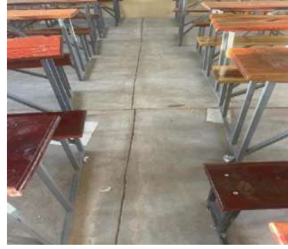
Expansion Gap not properly made
