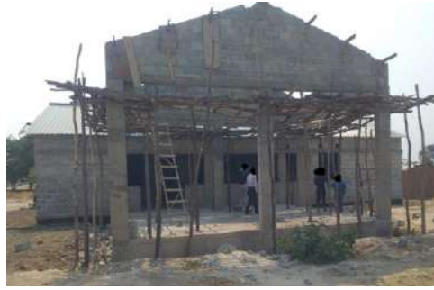
Incomplete Maternity Wing at Musele Health Post
