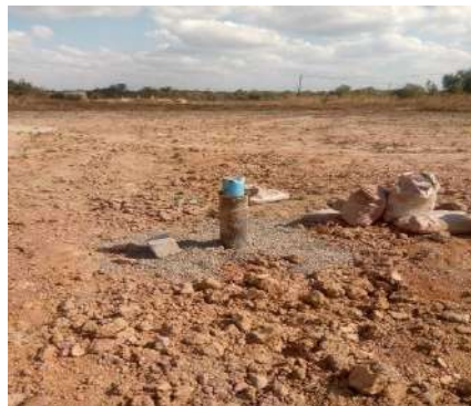
Uncomplete water reticulation system
