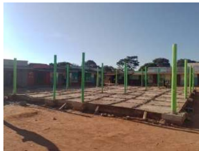
Incomplete market shelter
