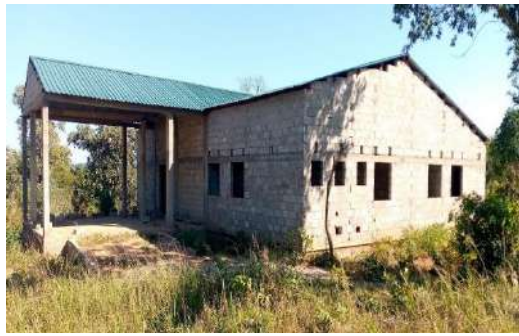
Incomplete Maternity Wing
