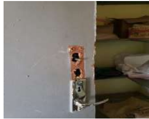
Broken mortice lock
