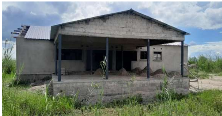
Incomplete Mung'omba Health Post
