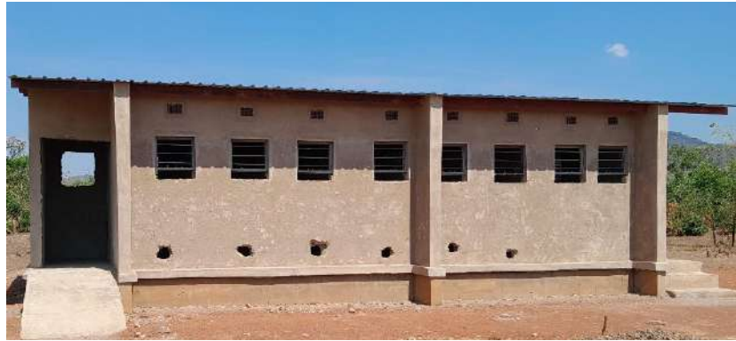
Incomplete ablution block
