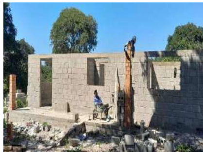
Incomplete maternity wing
