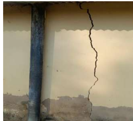
Dilapidated pit latrine being used
