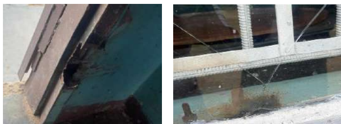
Door frame without a door Cracked window
