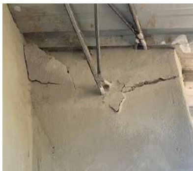
Cracked Concrete Padstone
