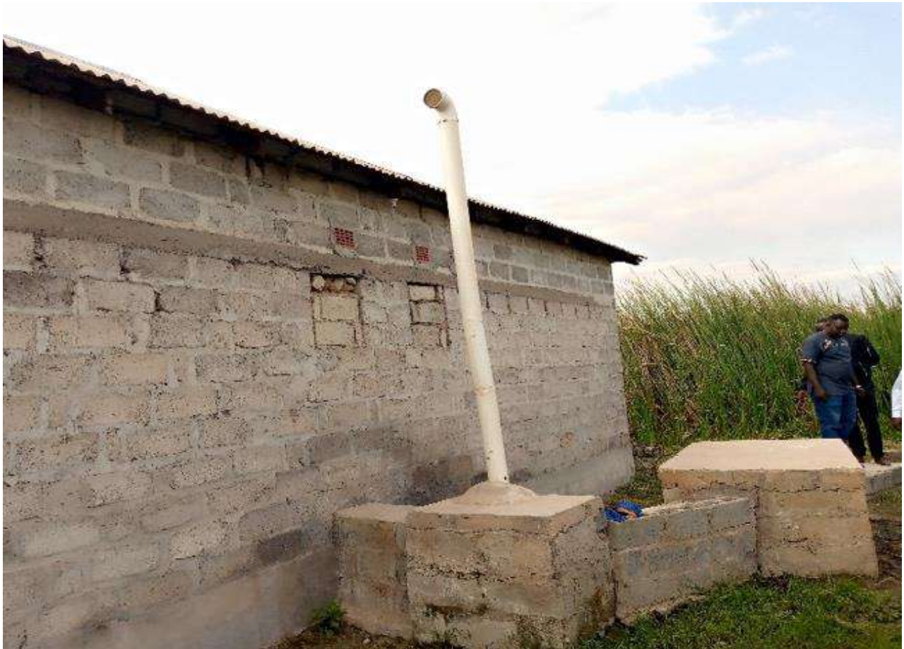
Figure 6.6(a): Septic Tank along the Riverbank - Source: Performance Audit –2022
