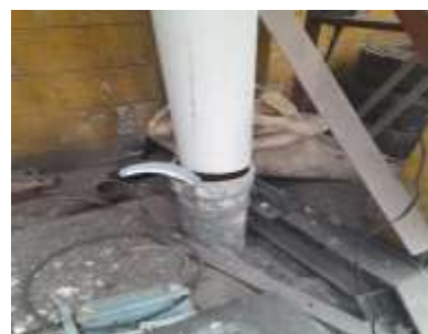
Incomplete Drain pipes
