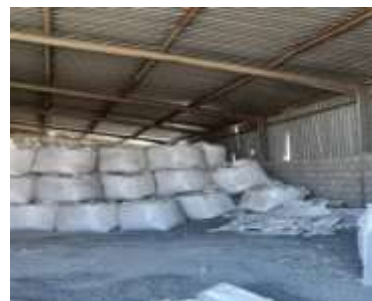
Warehouse number 5 in a poor state
