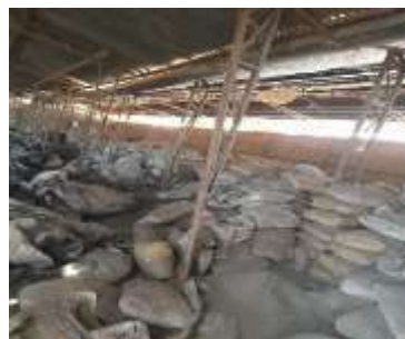
Dilapidated warehouse number 4
