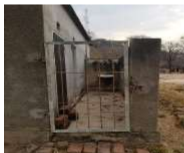
Dilapidated Toilet Structure
