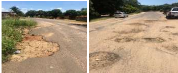
Potholes on Francis Town Road
