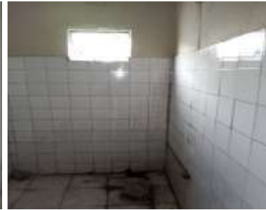
Bathroom with no shower
