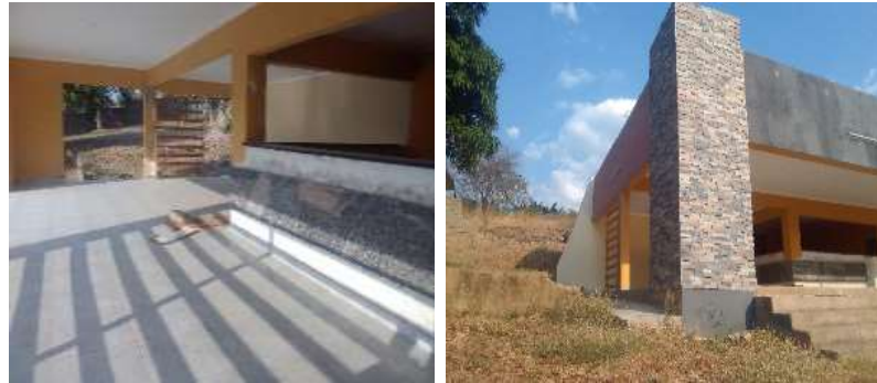
Part of the bar counter has not completely tiled. Electrical and plumbing works not completed
