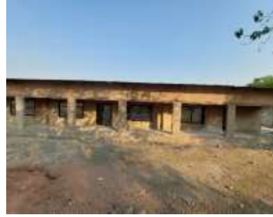
Fascia board and spoon drain around the structure not done
