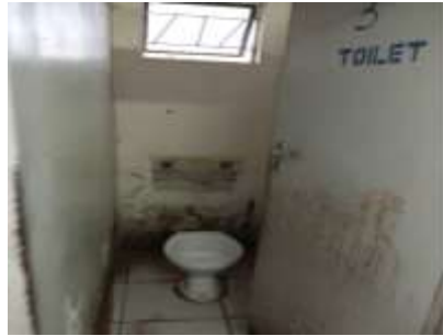
Toilet with no cistern
