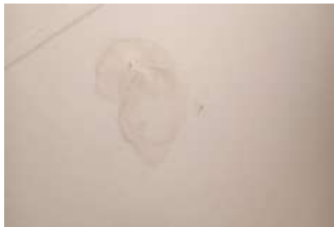
Leakages on the ceiling board
