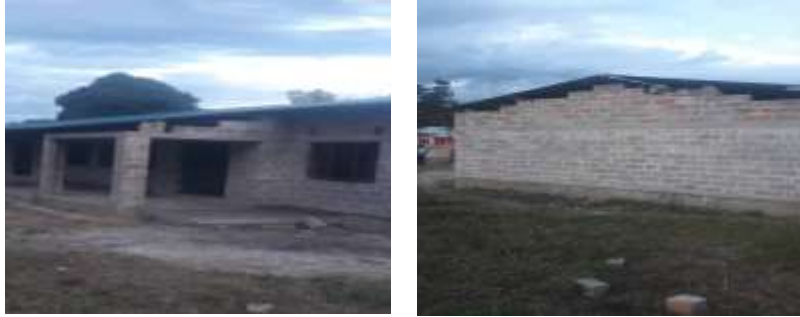
1x3 CRB at roof level at Beston Muluka Primary School
