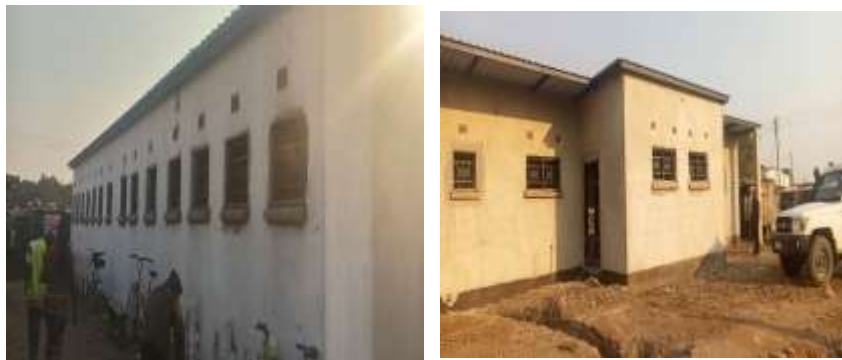
Incomplete Ablution Block at Chongwe Market
