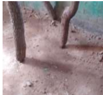
Floor Screed not Done
