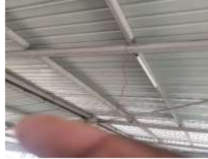
Vandalized Electric cables
