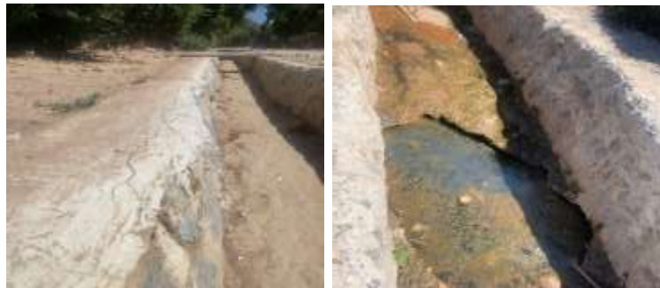
Cracks and small gully had started forming.
