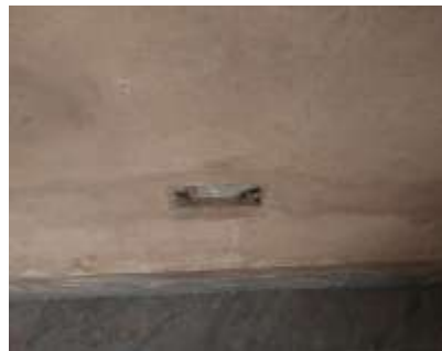
Socket not fitted
