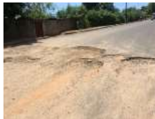
Potholes on Kombe Drive
