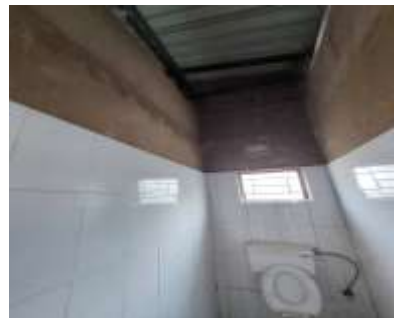
Ceiling boards in the toilets not fitted
