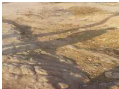
Gullies on Chibolya road
