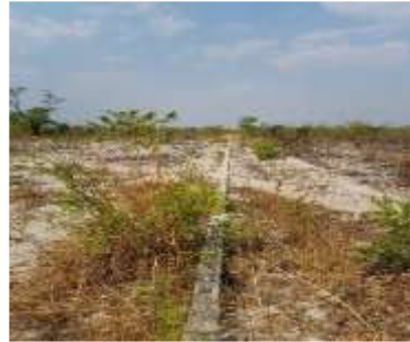
Incomplete Fence at the Dump Site
