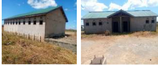
Incomplete Ablution Block at Wulongo Bus Station
