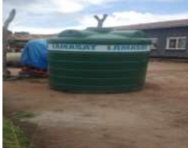
Water tank at council guest house
