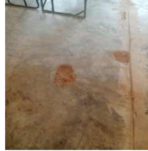
Holes and cracks – Classroom 2
