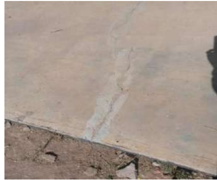
Cracks on the spoon drain
