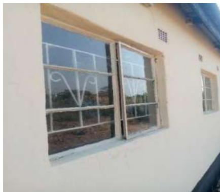
Window not closing properly
