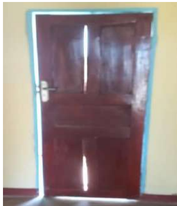
Poor quality door
