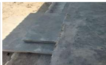
Cracked Staircase Floor
