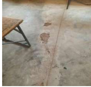
Holes and cracks – Classroom 1
