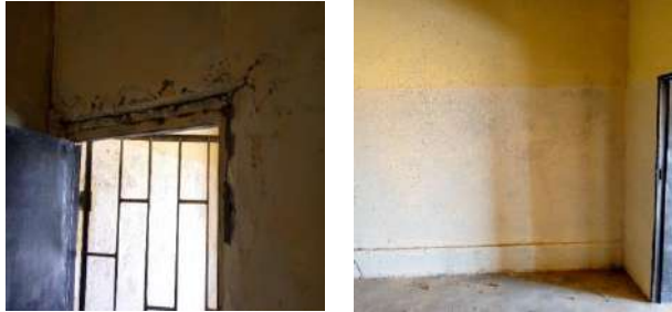
Rough and uneven plastered Surface-Interior part of the strong room
