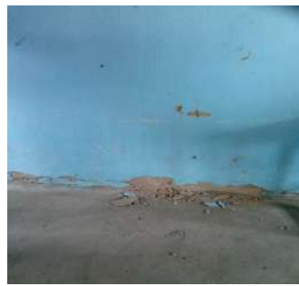
Plaster peeling off the wall
