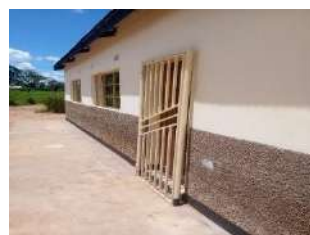
Grilled Door not Imbedded in Wall
