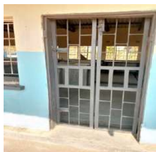
Glass panes and doors not fitted
