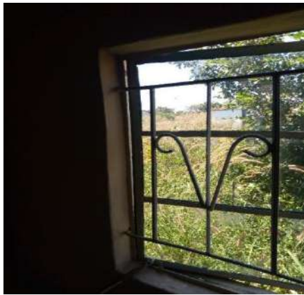
One side of the window failing off
