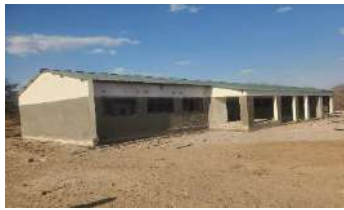
Incomplete 1x3 CRB at Machile Primary School
