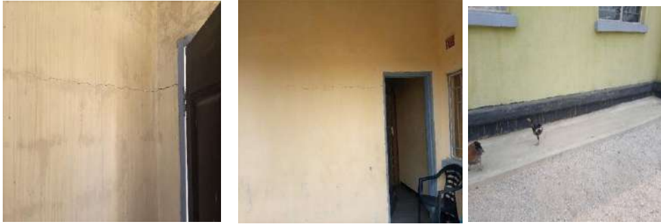
Cracked walls inside and outside the leaving room.
