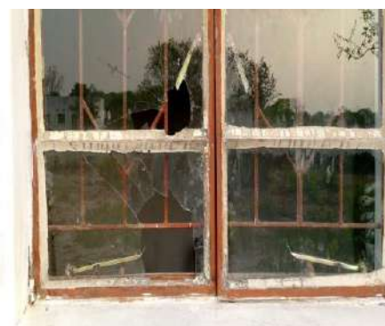
Broken windows at the Health Post
