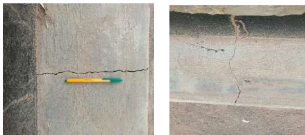
Cracks developing on the spoon drain
