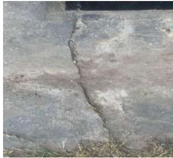
Cracks on Spoon drain
