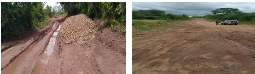
Incomplete Road in Simonga Ward
