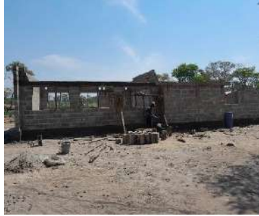
Delayed completion of 1x2 CRB at Mikube Primary School
