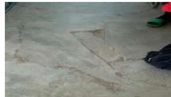
Cracks and potholes inside CRB
