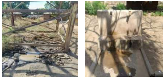
Formation of Mwalala Road and Culvert Installation in Mwalala Ward of Chama North
