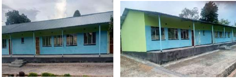
No Rough Cast on Blockwork
