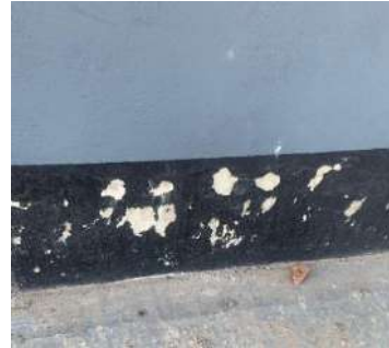
Paint peeled off
