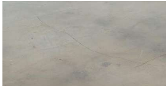
Cracks on the floor of the Classroom Block
