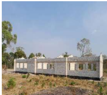
Delayed completion of 1x3 CRB at Mushokela
