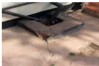
Poor workmanship on the galley and spoon drain
