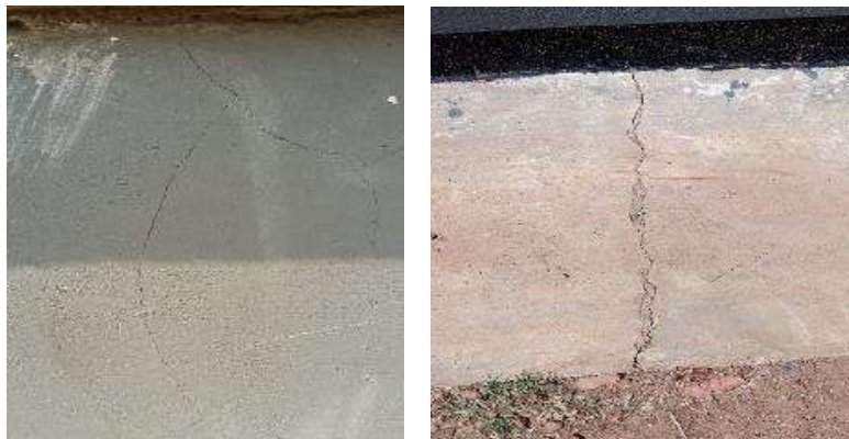
Cracks on floors, walls, aprons
