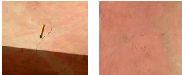
Cracks on the veranda and the floor
