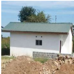
Incomplete wall fence
