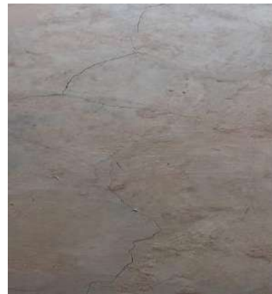
Evidence of cracks on floor
