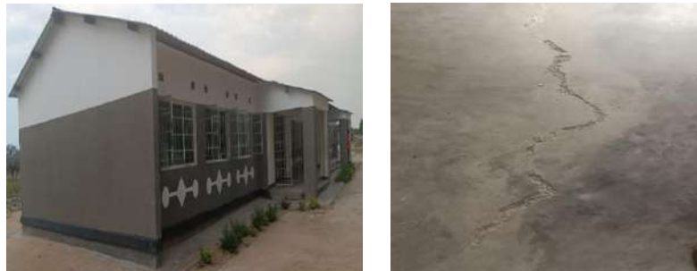
Cracks on the floor at Mupeta Primary School
