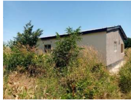
No electrification had been done
