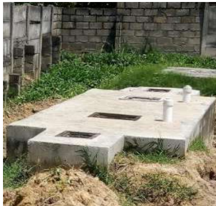
Manhole without covers
