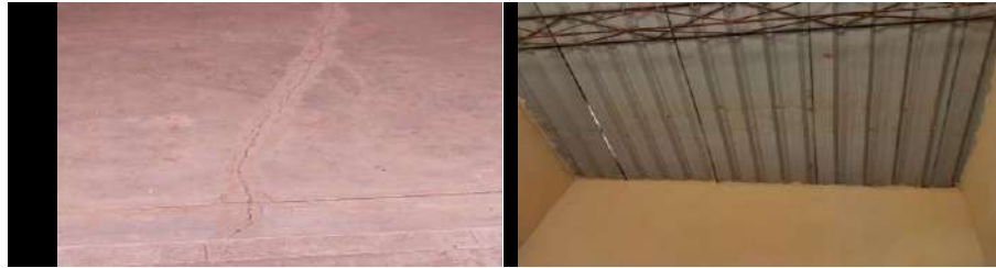
Floor with Cracks
