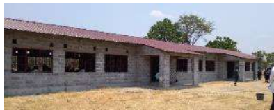
1x3 Classroom Block with Incomplete Works
