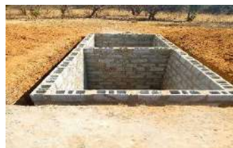
Delayed completion- Septic Tank at Makunka Primary School
