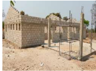
Delayed completion- Sikalai Health Centre
