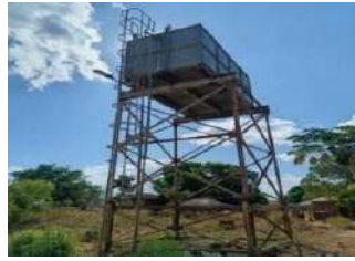
Defects on the Water Reticulation Scheme in Kambombo
