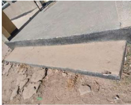
Poor workmanship on the step
