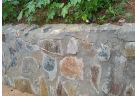
Cracks on the Compaction of the Lizuma Drainage
