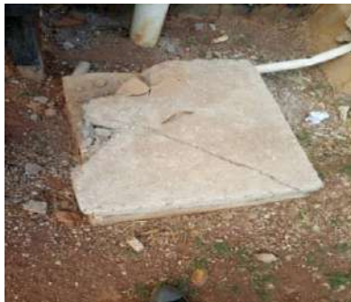
crumbling soak aways lids
