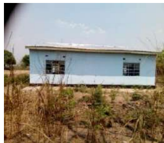
Roof with depression
