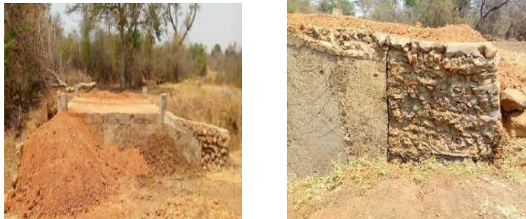
Partially done bridge with cracks
