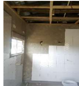
Ceiling not done
