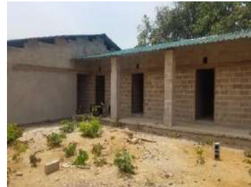
Floor and plastering not done
