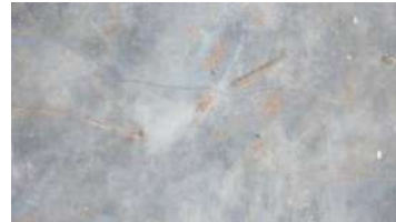
Cracks on classroom block
