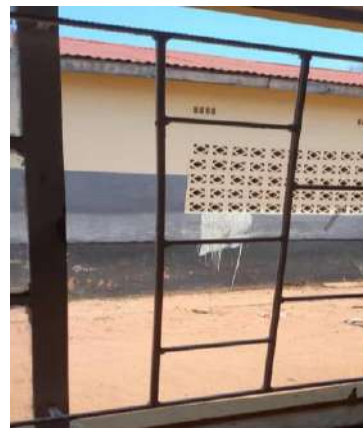
Window frame without window
