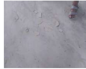
Floor peeling off
