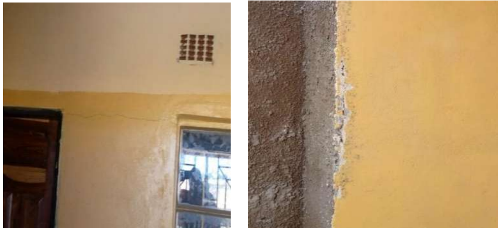
Cracks on the walls
