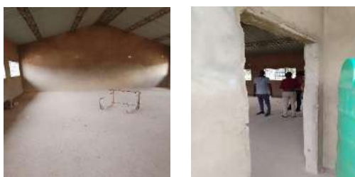
Unpainted and no floor screed laboratory and undone carpentry and iron mongery
