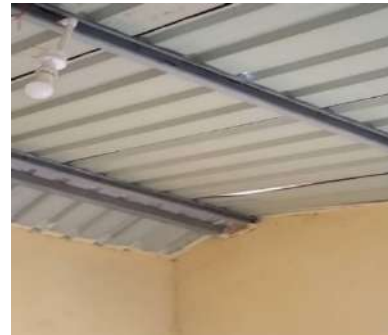
Leakages in the leaving room
