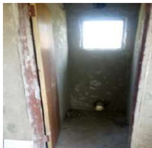
Plumbing not done
