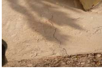
Cracks developing on the floor of the double VIP toilet
