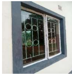
Window not closing properly
