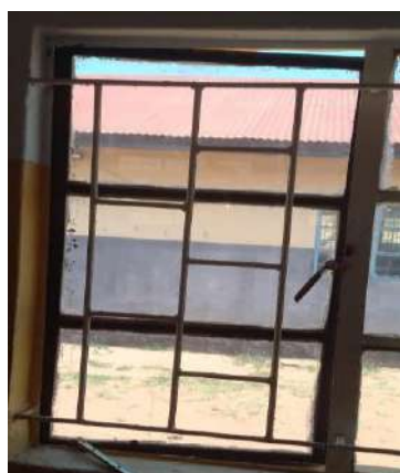
Poorly made window frame
