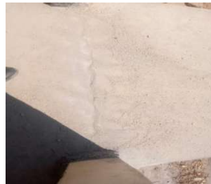
Poor workmanship on the veranda
