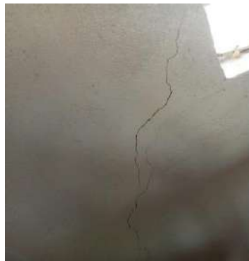
Cracks on the superstructure
