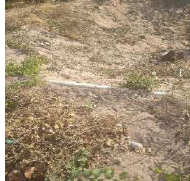
Exposed Sewer pipes
