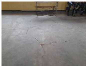
Cracking classroom floor
