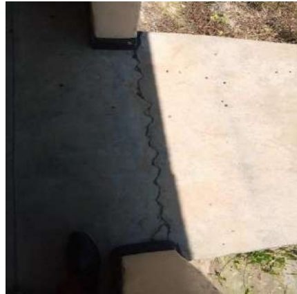
Crack on the veranda floor
