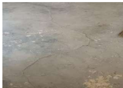
Cracks on the floor
