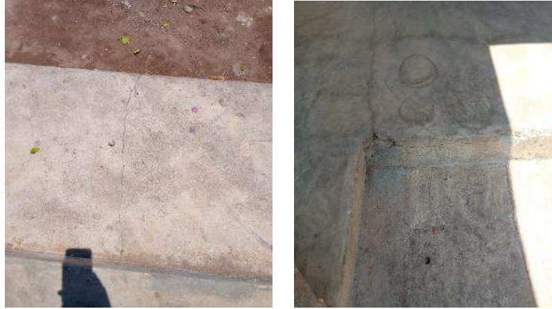
Cracks on the spoon drain and veranda
