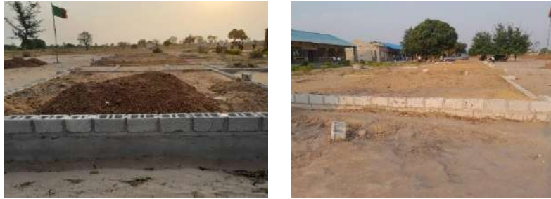
Stalled works at munkuye Secondary School
