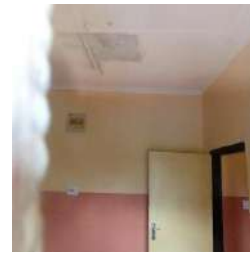
Stained Ceiling Board
