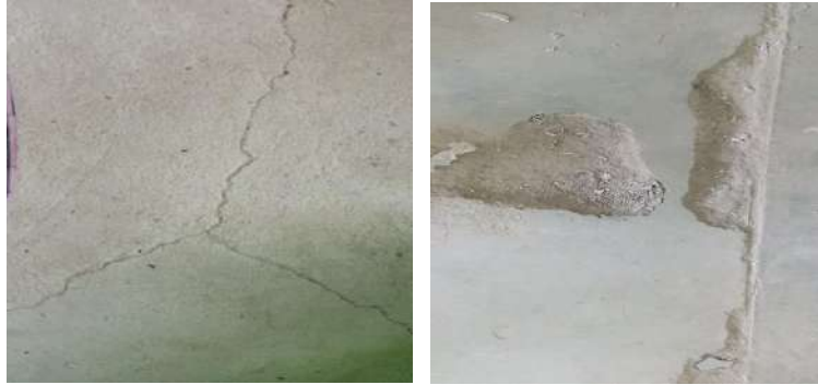
Cracked Spoon drain and Floor
