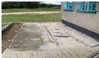
Cracks and potholes in spoon drain
