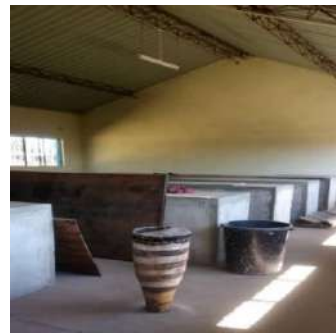
Uninstalled plumbing installations
