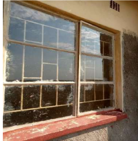
Window not closing properly
