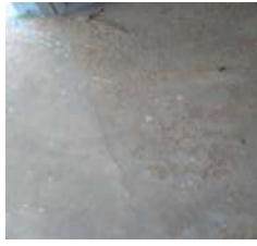
Hair Line cracks on the floor
