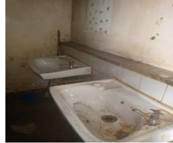
Dilapidated FTI – Sefula
