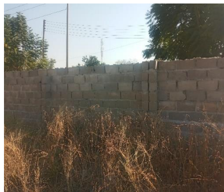
Loose block works
