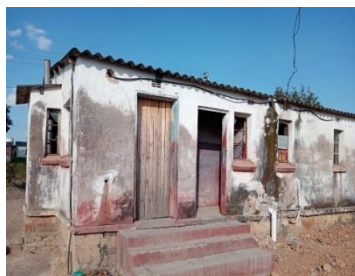
Outside Paint peeling off
