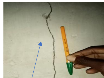
racked wall inside the house
