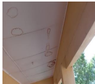
Leaking roof of the administration block
