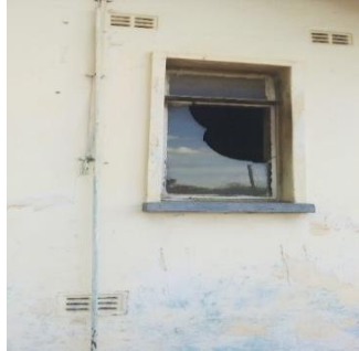
Broken glass window panes
