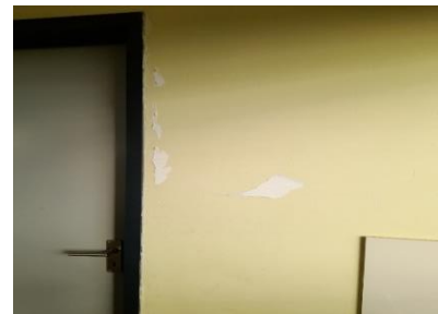
Peeling off paint at Msenga mini hospital
