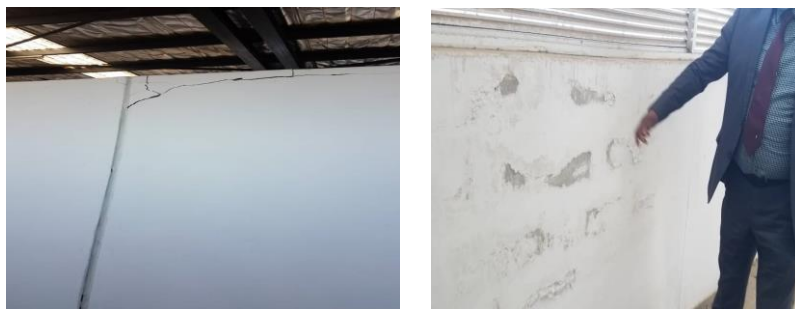
Cracks on the newly constructed walls and paint peeling off on just painted
