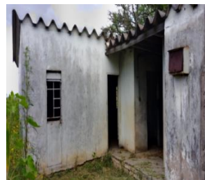
Dilapidated Servant Quarter at the DC's Residence
