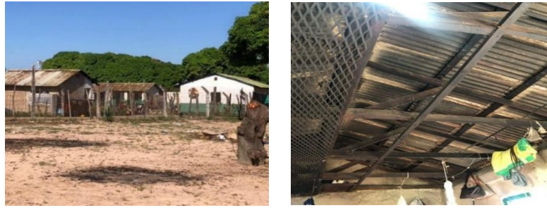
Partial wire gauze and worn-out wire fence
