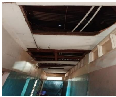
Fallen ceiling board
