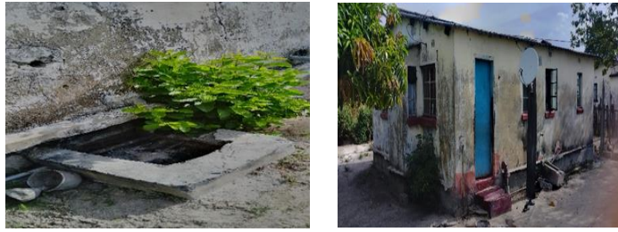
One of dilapidated Staff House and Sewer leakage at Namwala Correctional Facility
