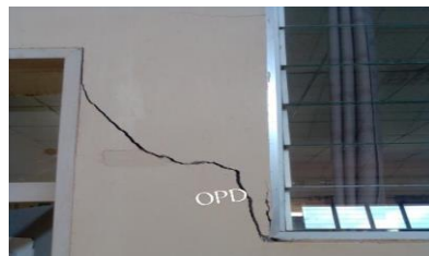
Crack on the wall of Out - Patient Department (OPD)
