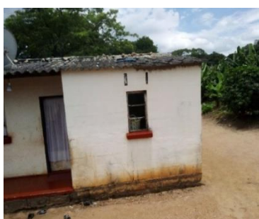
Dilapidated Low-Cost House
