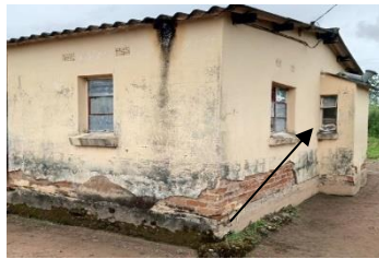
Dilapidated House and Broken Windows
