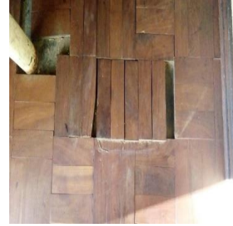
Damaged floor tiles
