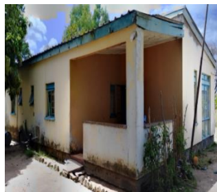
Dilapidated District Commissioner's Residence
