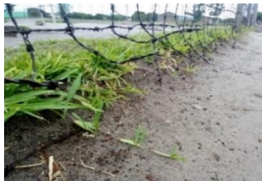
Unsecured Barbed Wires
