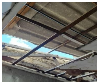
Blown off Roof and Worn out Ceiling
