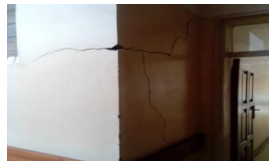
Cracks on the wall of Administration Block
