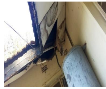
Rotten Ceiling Board
