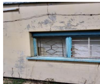
Visible cracks and broken window panes DC's Residence
