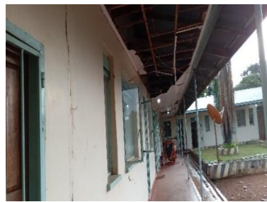
Administration block with damaged ceiling board and cracks
