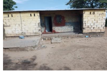
Dilapidated House – Chirundu
