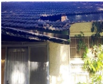
Worn out roof tiles
