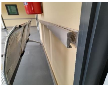
Broken fittings/wall at Milima mini hospital
