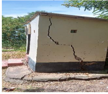
Crack on the VIP Latrine
