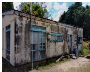
Rear View of dilapidated DC's Residence
