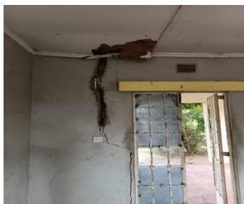
Crack inside the Labour Office
