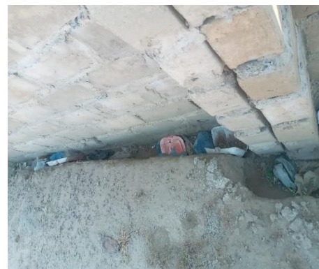
Foundation excavation not fully backfilled
