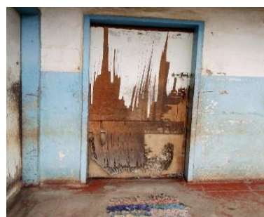
Worn Out Door
