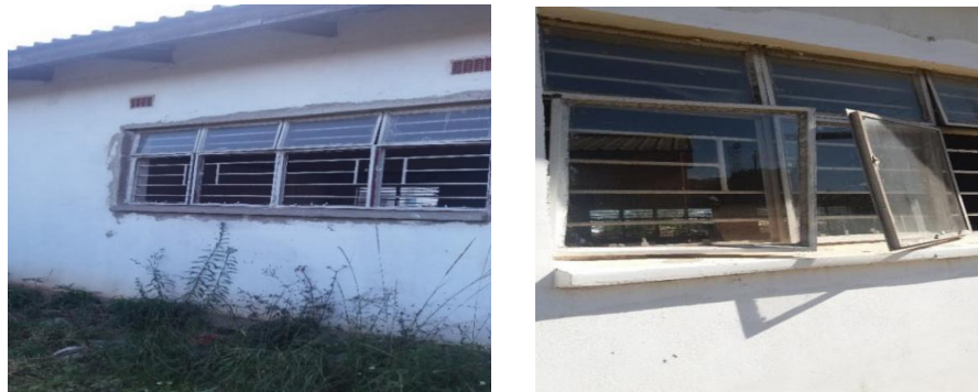
Figure 8.8: Missing Window Panes Stolen and Loose Window Frames almost Falling off
