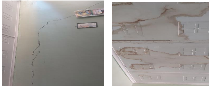
Figure 13.8: Cracks in the Wall and Leakage Marks on the Ceiling
