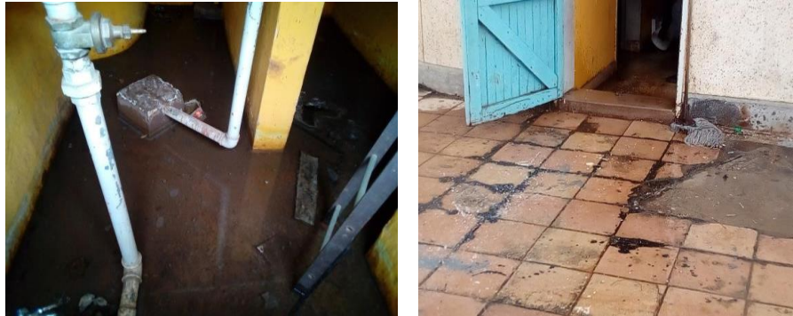
Figure 13.4: Leaking pipes on overhead tanks and damaged bitumen surfacing
