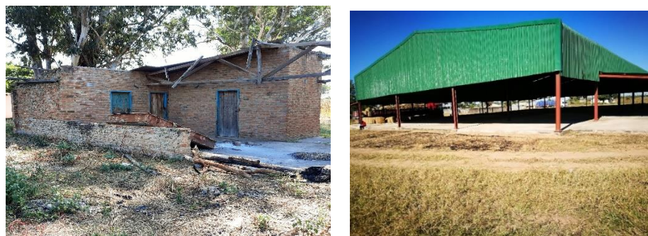
Figure 18.2: Dilapidated Office Block in Choma District and Incomplete Shed in Lundazi District
