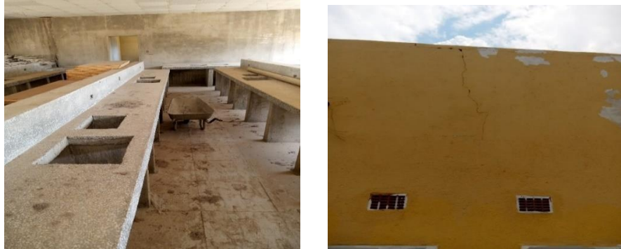
Figure 9.3: Incomplete Works Inside the Laboratory and Crack on the Wall
