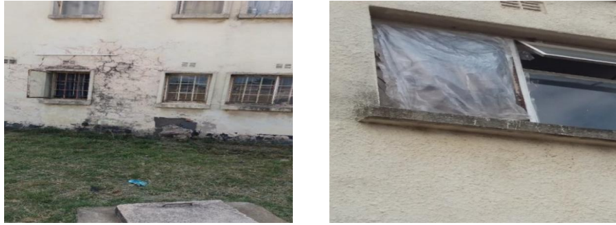
Figure 8.2: Cracked, Peeling off Walls and Broken Window Pane
