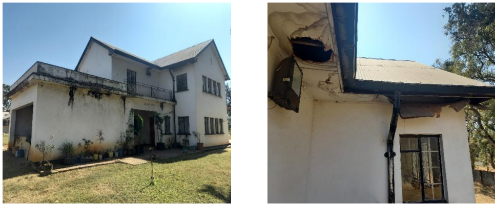
Figure 8.3: Poorly maintained Judges Residence with Damaged Ceiling due to Leaking Roof
