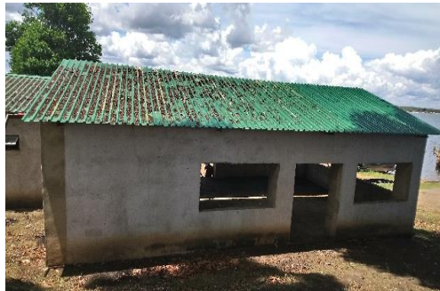
Figure 4.2: Incomplete waiting shelter
