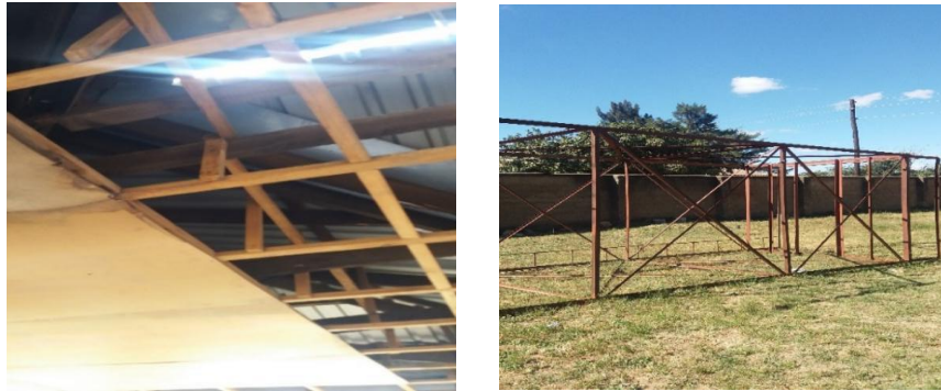
Figure 8.7: Ceiling Board not Completely Fitted and Uninstalled Tank Stand on the Ground
