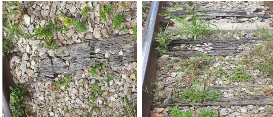
Figure 23.2: Rotten Hard Wood Sleepers over 30 years old between Lukanda and Walamba Area
