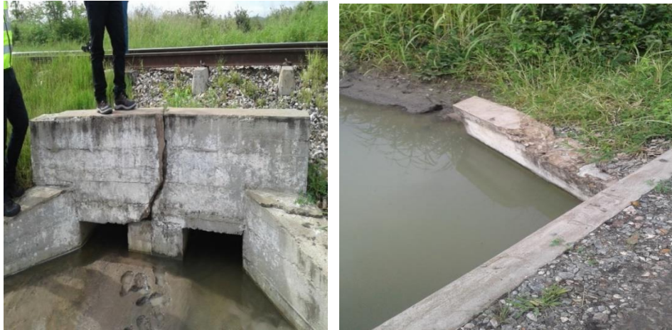
Figure 23.3: Cracked Culverts at Nega Nega and Luwombo Area
