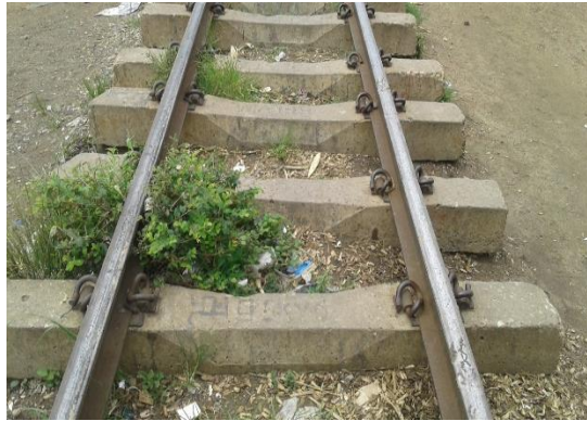
Figure 23.1: Lack of ballast along the rail line between Kamwala and Lilayi Area
