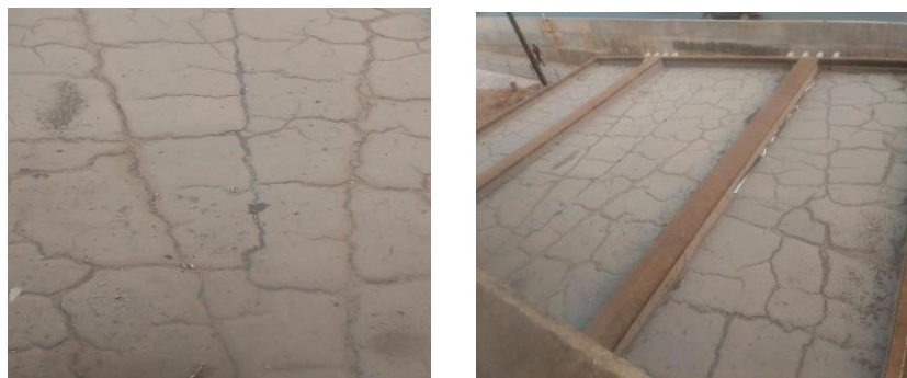
Figure 13.1: Cracked and Leaking Roof Surfaces
