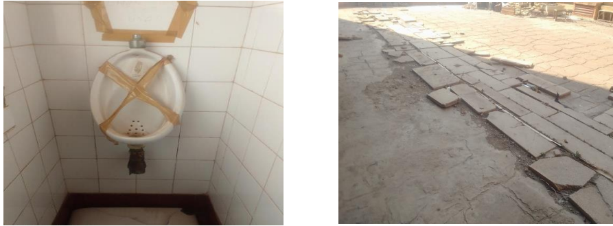
Figure 13.2: Obsolete Urinals and Cracked Bitumen Surface
