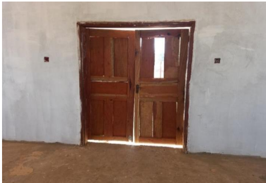
Figure 8.6: Fitted Double Doors with Visible Gaps
