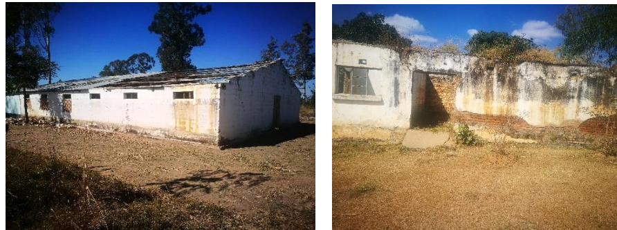
Figure 18.1: Dilapidated Structures in Chipata and Sinda Districts
