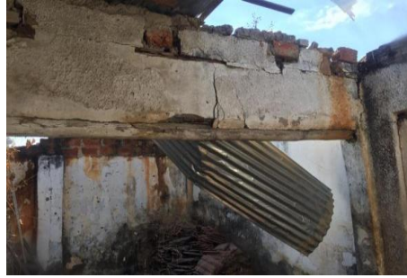
Figure 8.4: Collapsed Wall at Servant Quarters
