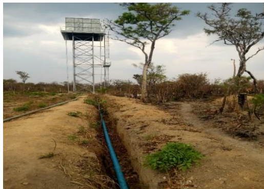
Figure 9.4: Pipe not Buried
