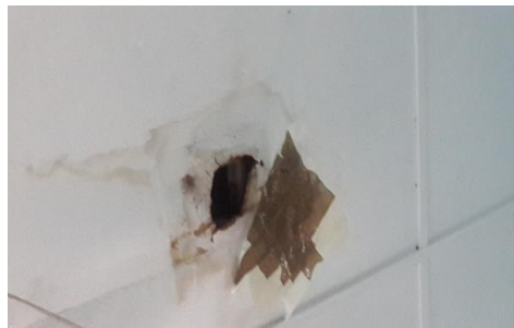
Leaking roof during rainy season
