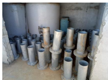
Parts of Modular plant laying unsecured
