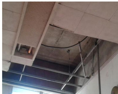
Damaged Roof in the ZNBS banking hall
