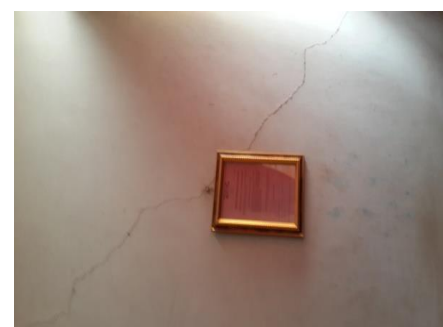
Cracks in the wall
