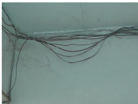
Dangling power cables
