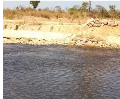
Floor of spillway being eroded falling on the spillway
