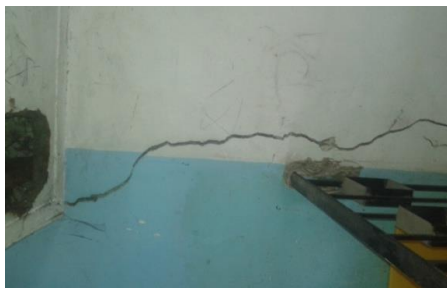
Cracks in the staircase
