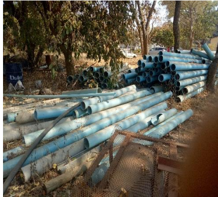
Some of the excess UPVC pipes exposed to adverse conditionalities
