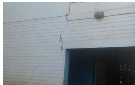
Cracks outside the building
