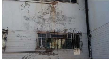
Gutters falling off
