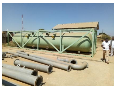
Un- assembled parts of the compact Modular Plant
