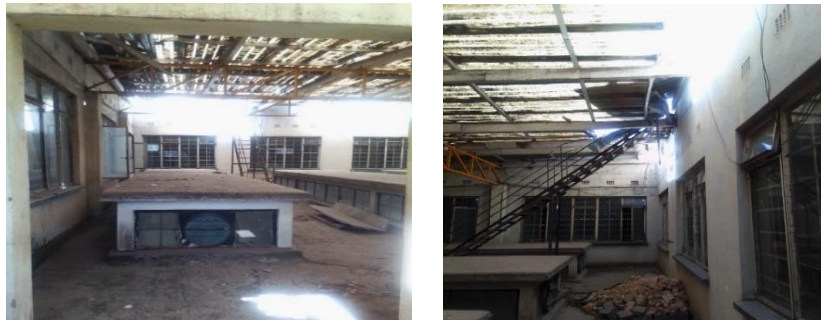
Dilapidated roof inside of Ndola Main Post Office earmarked for rehabilitation
