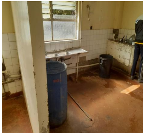
Worn out tiles
