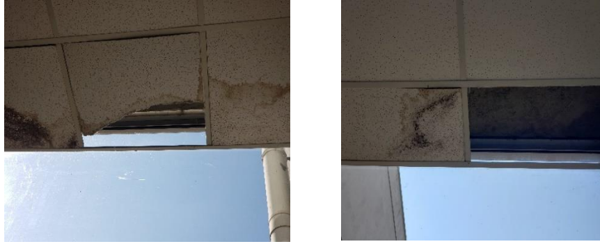
Stained and damaged ceiling boards
