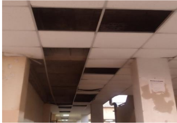
Dilapidated Ceiling – New Health Sciences Block
