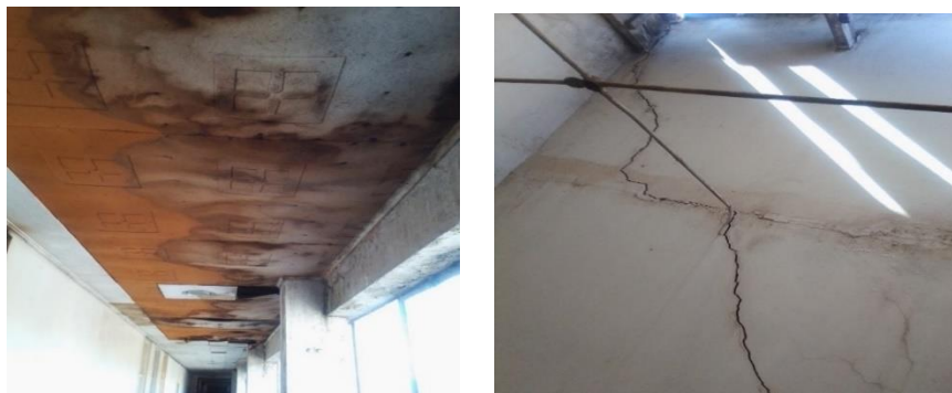
Stained Ceiling Board and cracked walls inside of the Post Office earmarked for rehabilitation
