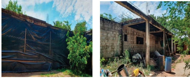
Picture 4.2: Abandoned Works at Chabanga Lodge-Solwezi
