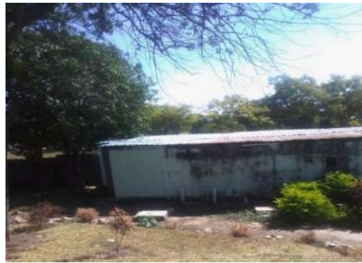
Ablution block not properly maintained
