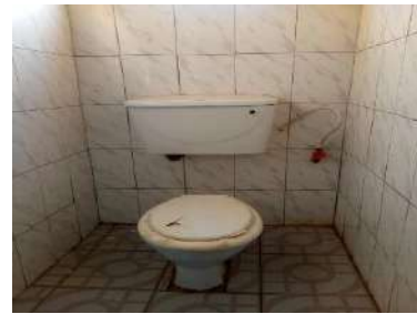
Non-functional cistern and broken toilet cover
