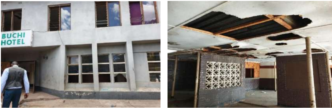
Dilapidated Buchi Hotel
