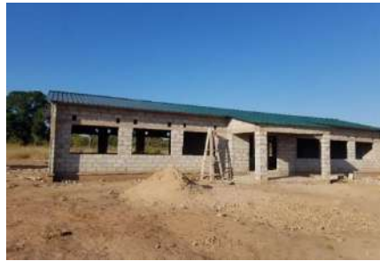
Incomplete 1x2 CRB at Mabombo Primary School
