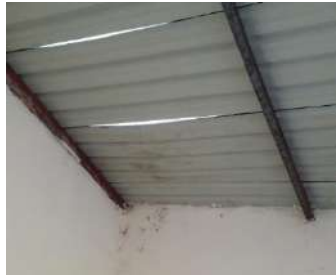
Spaces between iron sheets
