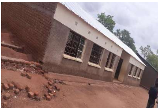
Incomplete 1x3 classroom block
