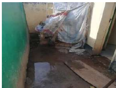
Dirty entrance at the main market toilet
