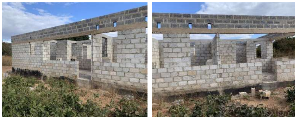
Incomplete clinic at Chipapa
