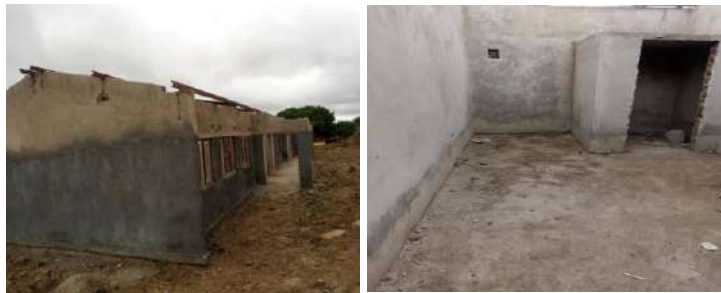
Incomplete 1x3 CRB at Kampishi Primary School
