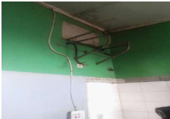
Missing geyser -swimming pool kitchen
