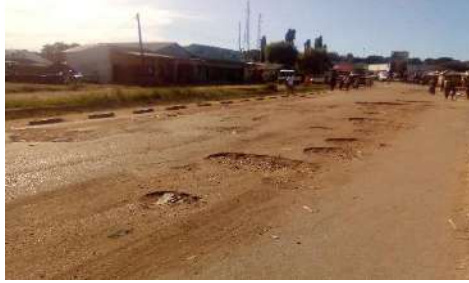
Potholes along Mpulungu - Mbala Road
