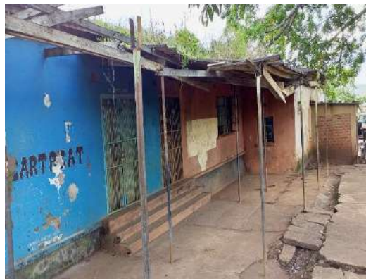
Dilapidated Council Bar
