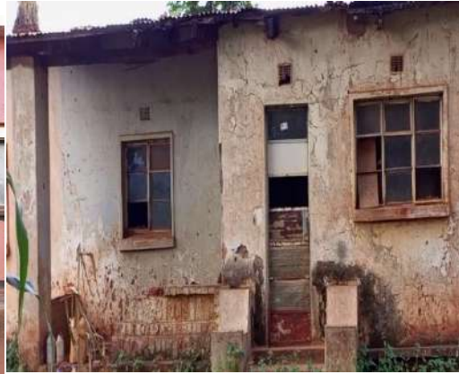
House No. 2 Abandoned house
