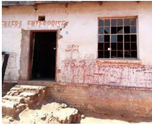
Shop with broken glass panes
