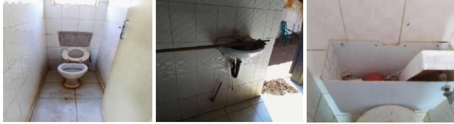
Non-functional cisterns and sinks in the ablution block
