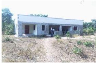
Incomplete Health post
