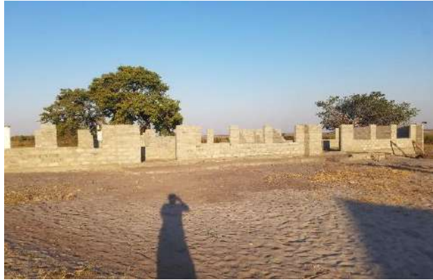
Mataba Primary School - Stalled Works
