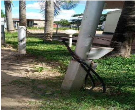
Cables cut from the pole - Almalik Road
