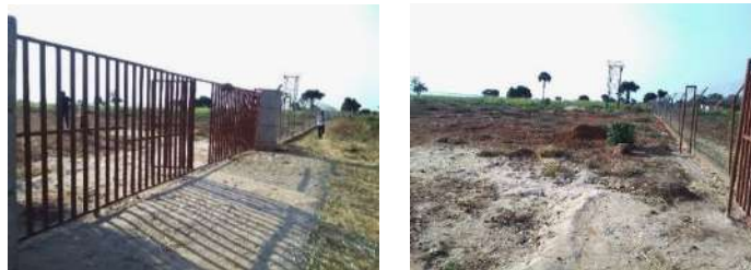
Incomplete Truck packing bay
