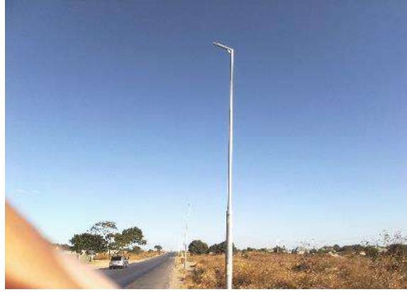
Vandalized street light
