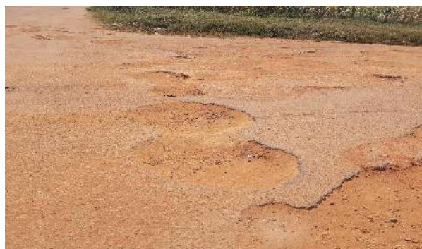
Potholes along Market Road
