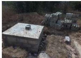
Incomplete VIP toilet
