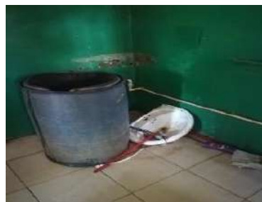
Broken Sink at the main market
