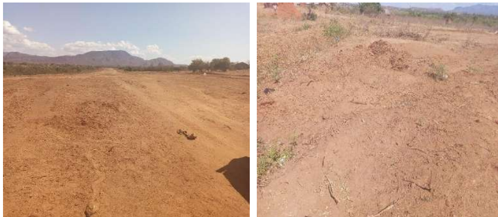
Uneven surface of the graded runway of the Airstrip
