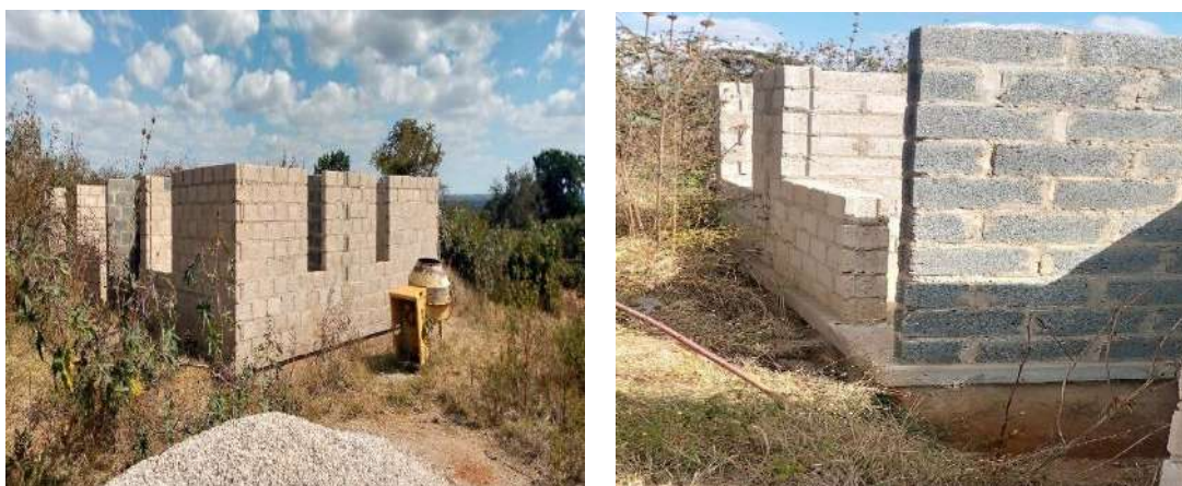
Incomplete staff house at Hapwaya Clinic
