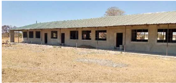
Incomplete 1x3 classroom block.
