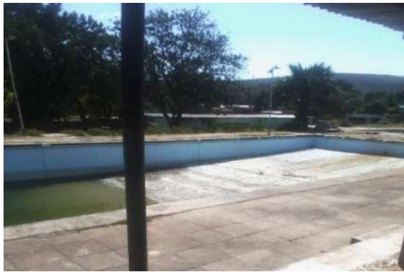
Swimming Pool not maintained
