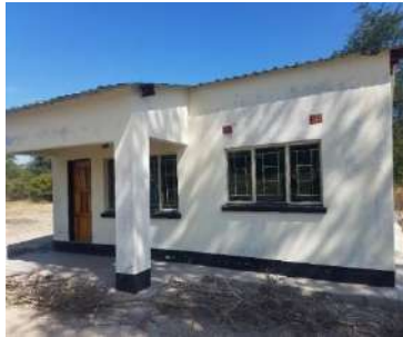
Once painted walls peeling off at Sikuze.
