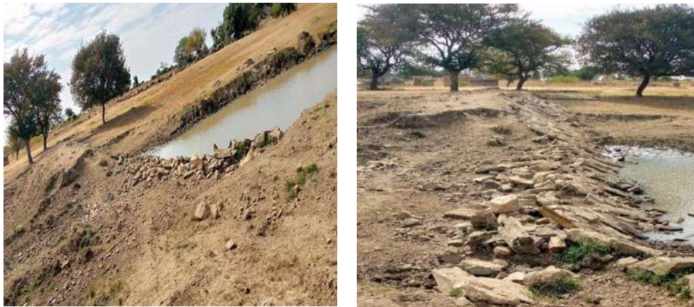
Eroded embankment of the weir dam
