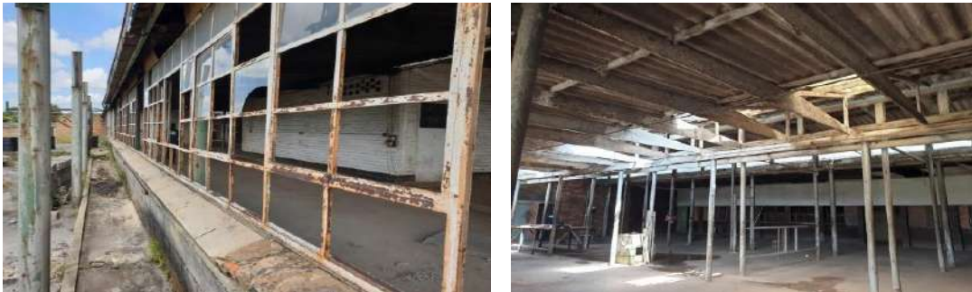
Dilapidated Bamboo Building Workshop
