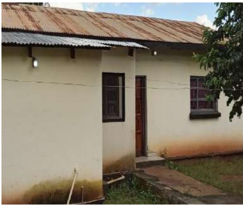
House No. 3: House with corroded roof
