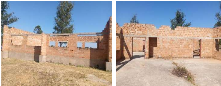
Stalled Project at ring beam level with some portions at gable level
