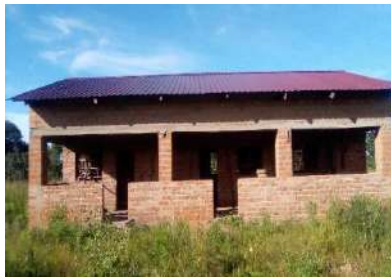
Incomplete Nakalengule Health Post
