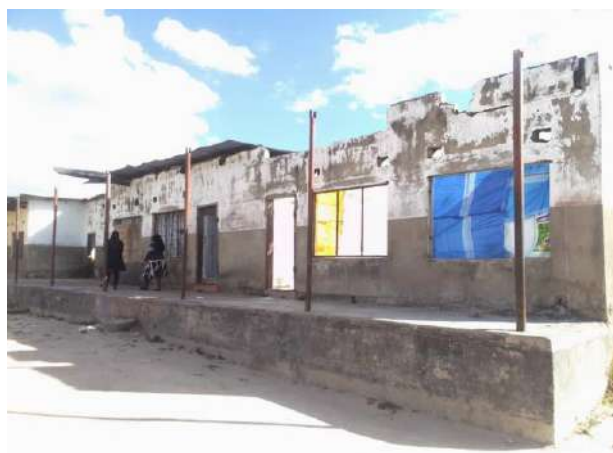
Dilapidated Push hall
