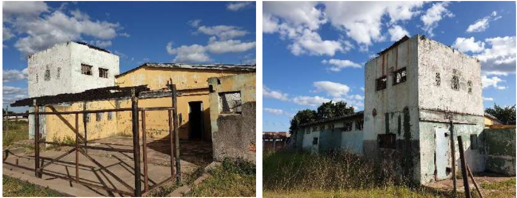
Dilapidated East Bar in Mikomfwa
