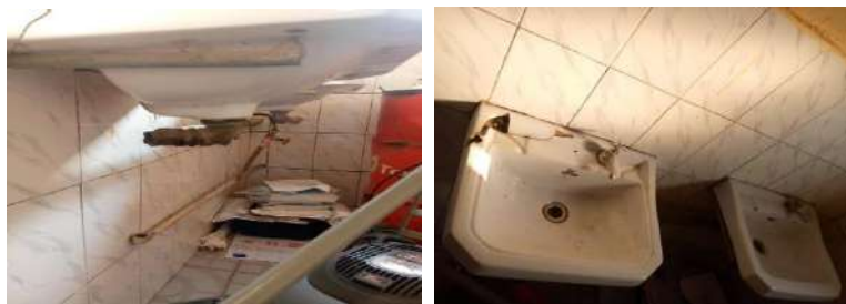
Non-functional sinks and taps
