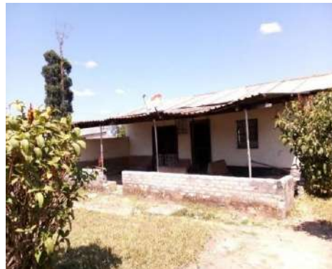
Warped roof in the Verendah
