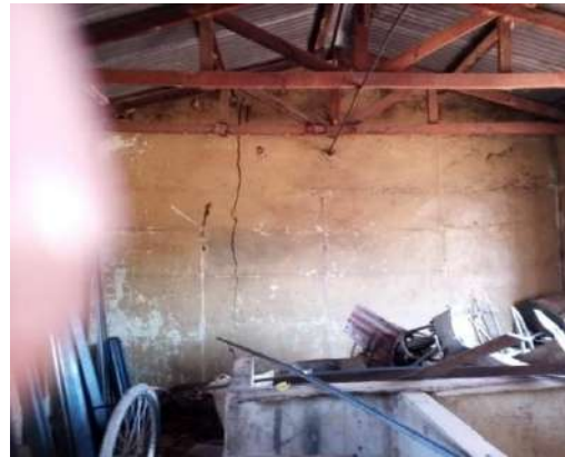
Cracks on the walls of the shop
