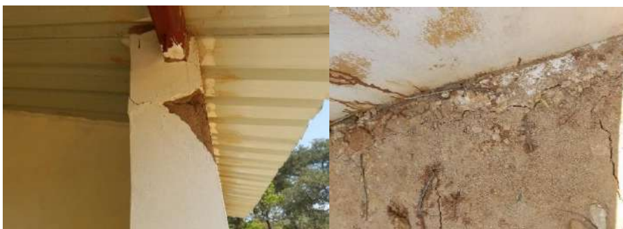
Cracked Walls to OPD
