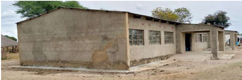
Incomplete 1x3 classroom block
