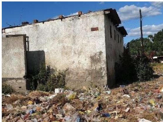
Dilapidated Ablution block at Mikofwa Main Market
