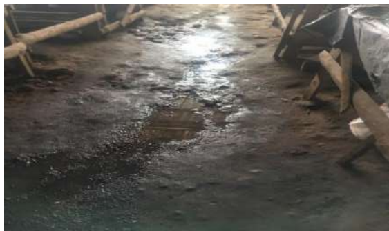
Chisokone Fish Shelter without concrete floor
