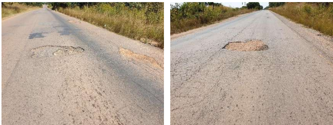
Poorly Rehabilitated Luanshya – Ndola Road
