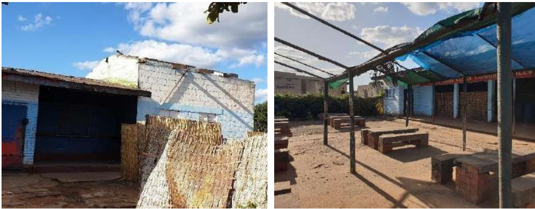
Dilapidated Muchinsi Cocktail Bar
