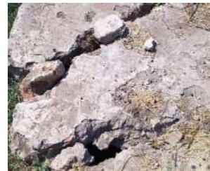
Broken Septic Tank
