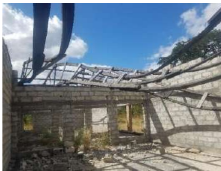
Trusses falling on the unroofed part
