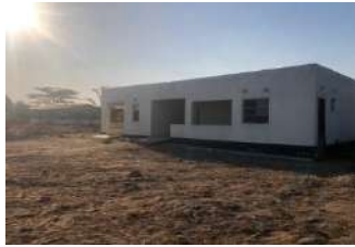
Incomplete Health Post
