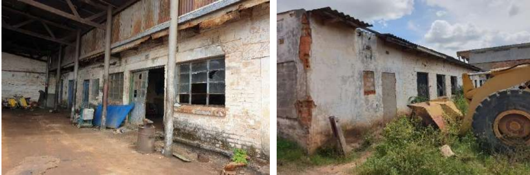
Dilapidated KMB Mechanical Workshop
