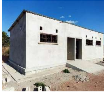
Incomplete Ablution Block
