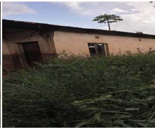
House No. 4: Abandoned house
