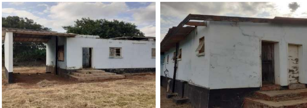
Dilapidated Motel Rooms
