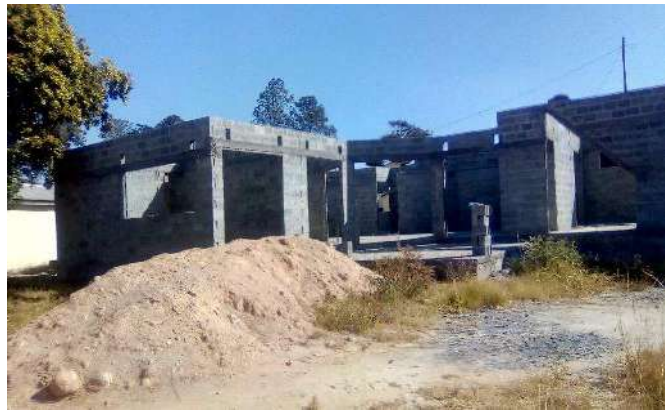
Incomplete Community Library
