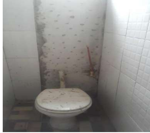
Incomplete wall tiling and fittings in toilets
