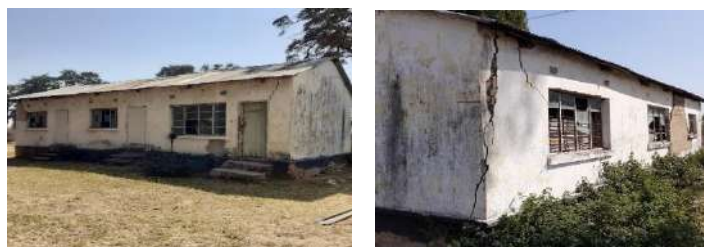
Dilapidated Old Stores Office
