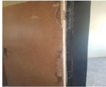
Flush doors eaten up by termite
