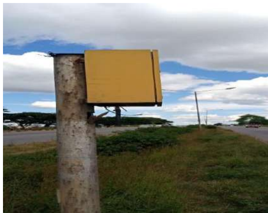
Vandalised pole and Electric Cables
