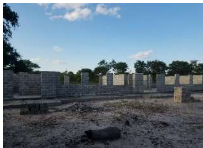
Incomplete 1x3 CRB at Sibukali Secondary School
