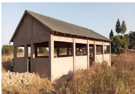
Incomplete market shelter at Bweupe
