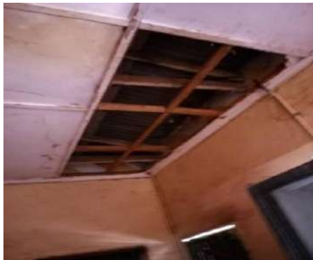
Partially fallen Ceiling board
