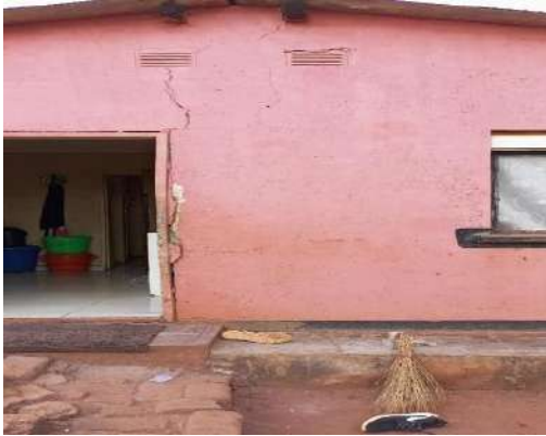
House No. 1 with a crack
