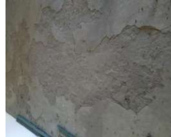
Cracks on the floor
