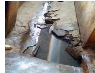
Stagnated water in the corridor
