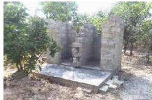
Incomplete VIP toilet
