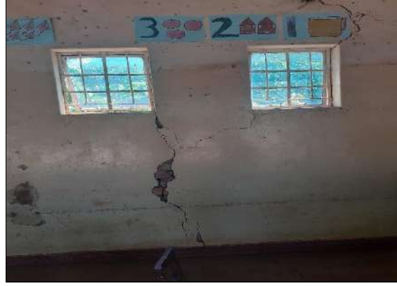
Dilapidated Libuyu Community Hall
