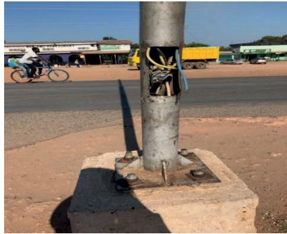
Vandalised street light pole
