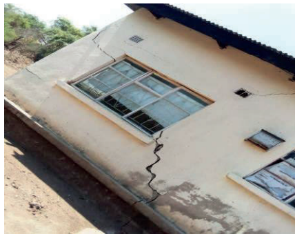
House No. 1473 had a crack in the corner and through a room
