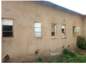
Broken windows and holes in rooms
