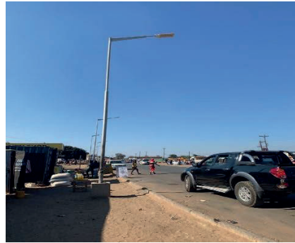
Street lights along the Great East Road
