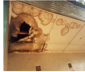
Damaged Ceiling – Nchete Guest House
