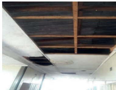
Ceiling board in corridors at Finance Department
