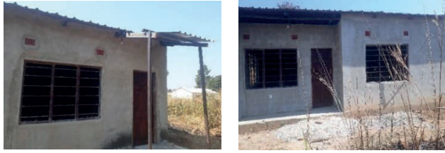
Incomplete Construction of a Staff House
