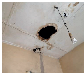
Damaged Ceiling Board
