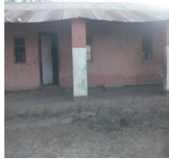
Dilapidated Council House
