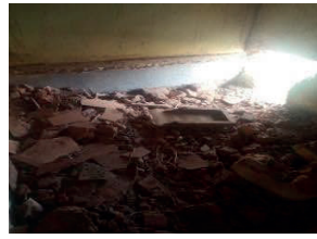
Debris inside the rooms
