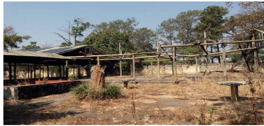
Blown off roof - Court yard
