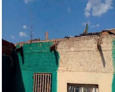
Scrapped off roof of the Restaurant
