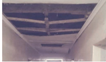
Broken Ceiling boards
