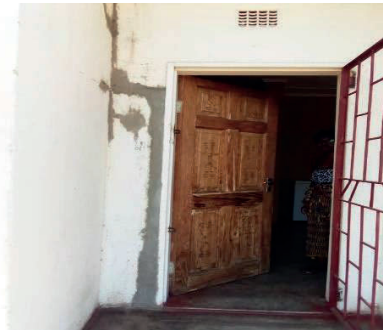
House No. 1475 cracks on the veranda had been mended, but painting still remained outstanding
