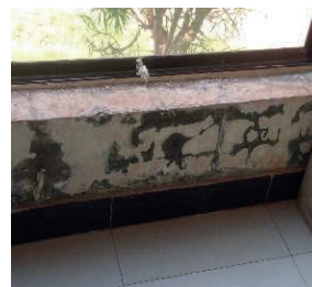
Wall tiles peeled off
