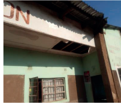
Dilapidated ceiling board
