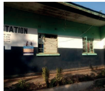
Dilapidated Police Station
