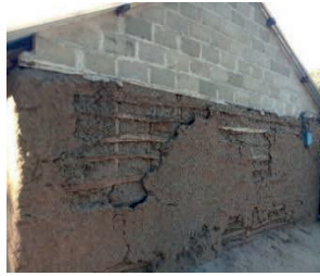
One of the five (5) houses plaster peeling off
