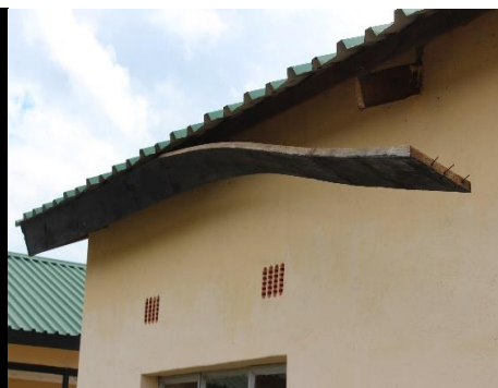
Poorly fitted board
