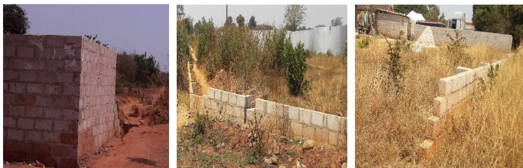
Abandoned construction of a wall fence
