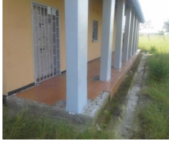
Fixing of floor tiles on veranda not completed
