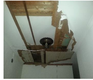
Falling Off Ceiling Board
