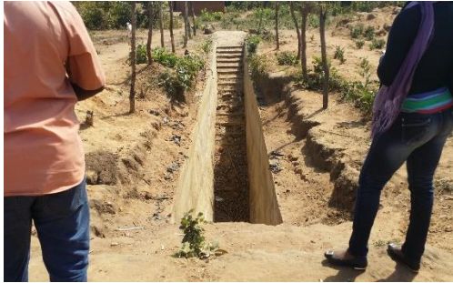
Nyampande Dip Tank not Done
