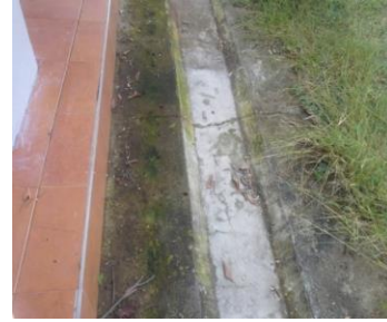
Cracks on the drainages
