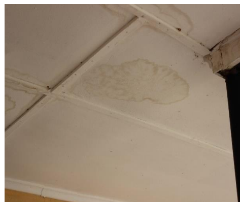
Leakage in one of the offices
