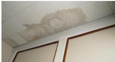
Stained ceiling in the Deputy High Commissioner's Office
