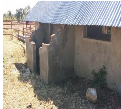
State of Kagoro Dip Tank
