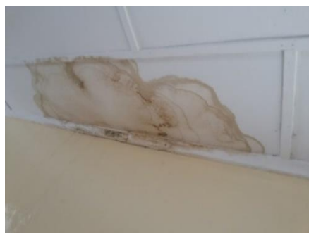
Stained ceiling board due to leaking roof
