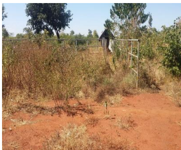
Incomplete Works at Kalichelo Dip Tank
