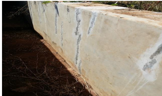
Wall Needs Attention to Mend Cracks
