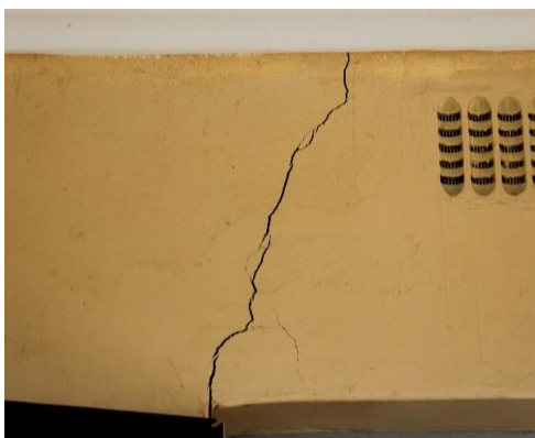
A crack on the wall
