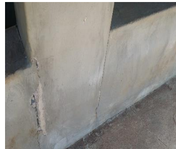
Cracks on Walls of Chiparamba Dip Tank
