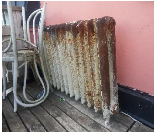
Unserviced Heating Radiator
