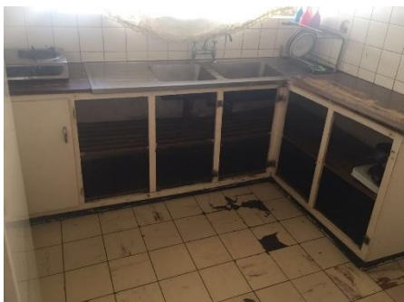
Damaged kitchen unit
