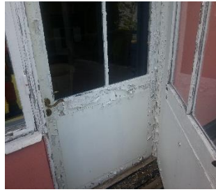
Peeling Paint on Doors
