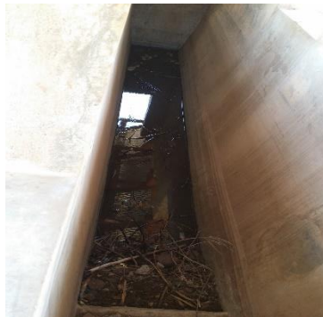
State of Kagoro Dip Tank
