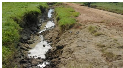
Eroded road due to deviation culvert not removed
