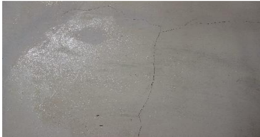
A crack on the wall of the Labour office
