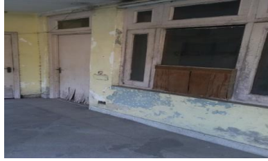
Dilapidated Back entrance at the old residence
