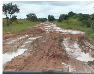
Road deformed and sinking at 12.3km
