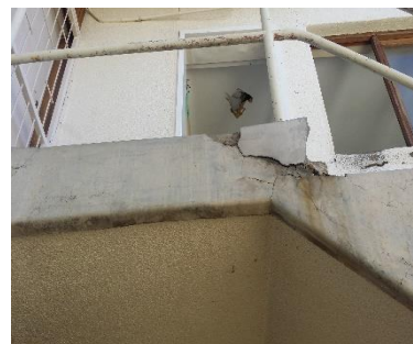
Broken stair case
