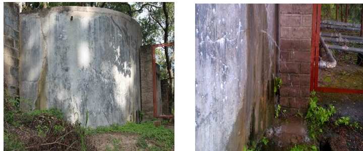
Cracks developing on the walls of the rehabilitated reservoir and water leaking due to poor workmanship
