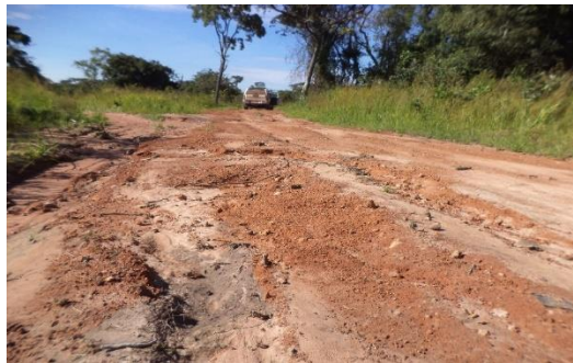
At 8.7 km road eroded
