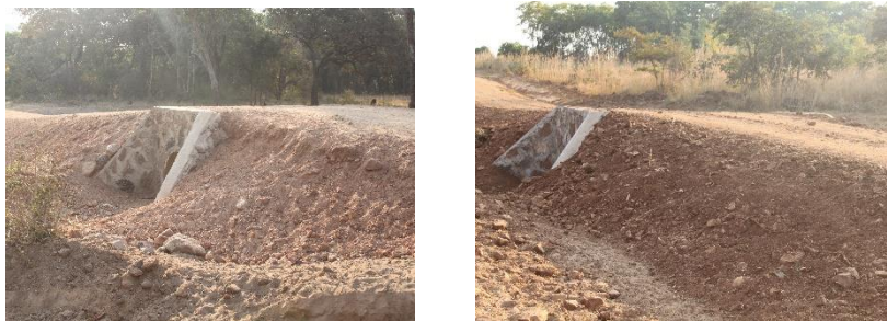
Embankments at chainage 8.9 km and 13.8 km poorly compacted and being eroded
