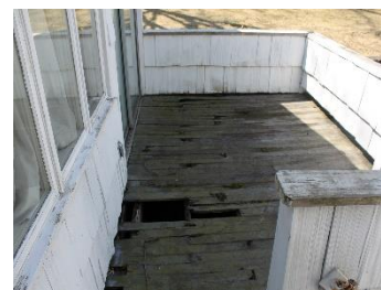
Rotten wood panels on the veranda
