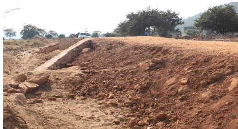
Embankment of the culvert at chainage 5.7 km poorly compacted
