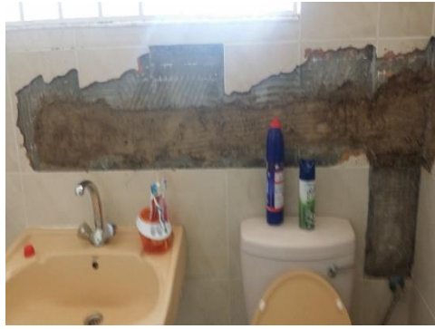
Wall from which tiles were removed
