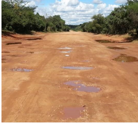
Silted culvert at 4.0km Nampundwe Rd
