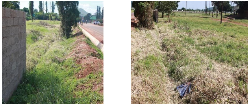
A foundation trench measuring 59 metres excavated without block work at the abandoned DK Stadium
