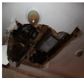
Rotten ceiling in one of the bedrooms
