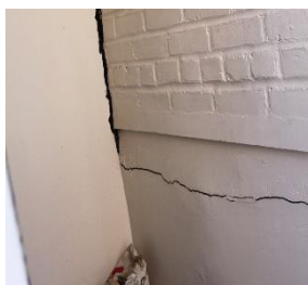
Cracked basement wall
