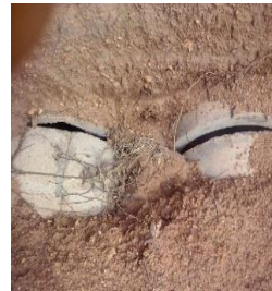
Exposed Culverts - Tara- Katete, Kalomo
