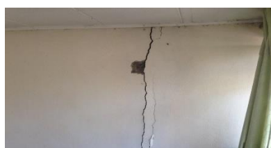
Crack in one of the offices
