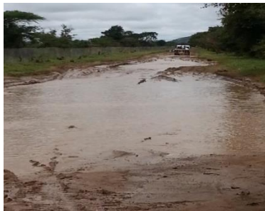
Depression and water ponding at 6km
