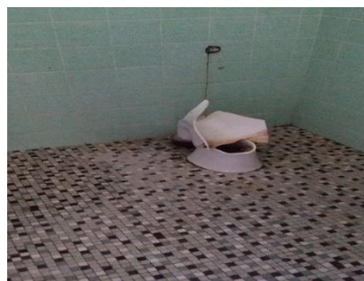
Vandalised Toilet Bowl
