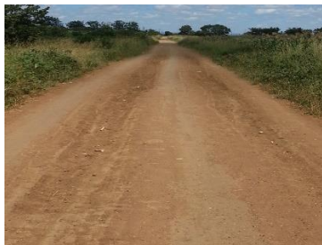
Wheel rutting at 8.6km
