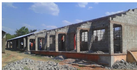
A 1 x 4 Class Room Block Partially Roofed at Anoya Zulu Secondary School
