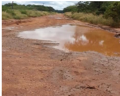
Water ponding at 20.9km Makeni rd
