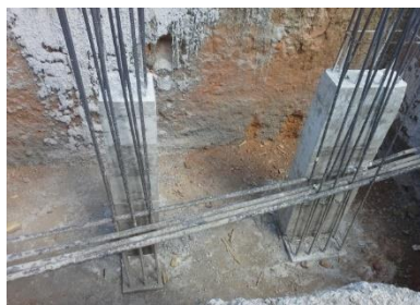
Power cables passing through the site
