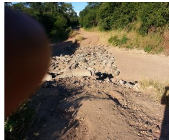
Washed away culvert at 3.7 km
