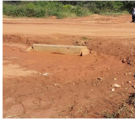
Pot holes and water ponding at 6.2km Nampundwe Rd.
