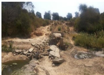
Collapsed Spillway at Mulobezi Dam
