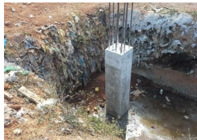
Garbage at the construction site
