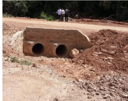
Inlet of the culvert with eroded debris on the upron
