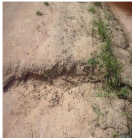
Gully across the road - Tara- Katete
