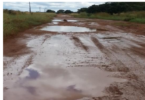
Depressions and water ponding at 22.4km Makeni rd.
