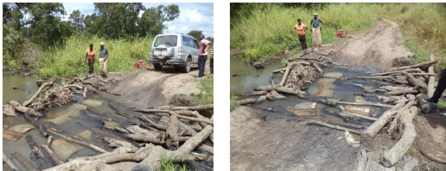
Culverts not installed at +7.2 km, a stream cutting across the road
