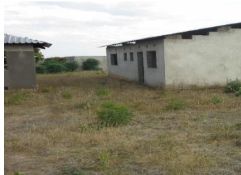
One of the abandoned houses
