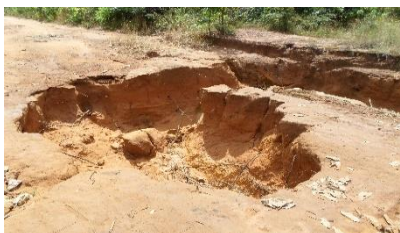
Portion of the Mwambashi Road eroded at 0.6 km
