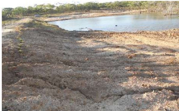
Soil erosion of the embankment formation of Chasato dam
