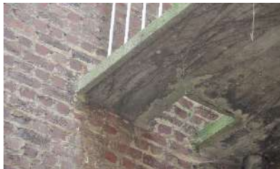
Cracks Underneath the Balcony
