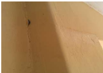
Crack on the wall
