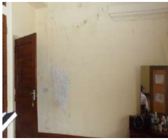
Seepage of water in the wall
