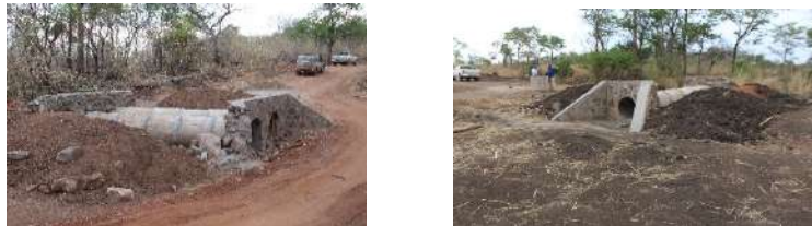
Double line culverts not buried on Mwape Road
