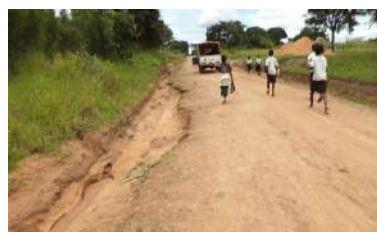
Eroded road due to lack of drainage
