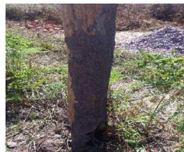
Untreated Poles attacked by termites
