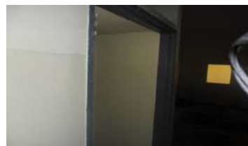
Door not replaced
