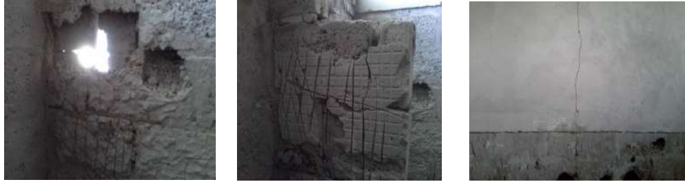
A hole created on the wall and weak walls in the Showers at the Intercity Bus Terminus in Livingstone
