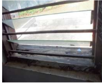
Falling off louvers
