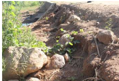
Embankment eroded on culverts at Chiuta River along Mwanjabantu – Mumbi Road
