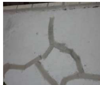
Mended roof chancery
