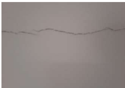
Cracks in the minor living room
