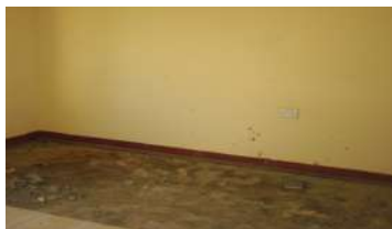
Incomplete Tile Installation
