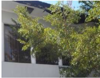
Ceiling board falling off at the balcony
