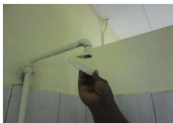
Defective Shower Rose
