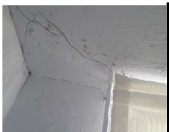
Crack in the Living room
