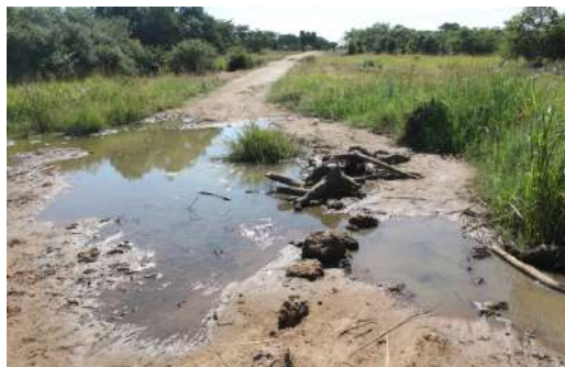
Water ponding on Mwanjabanthu – Nyanje road due to poor drainage
