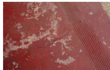
Paint peeling off on the Veranda
