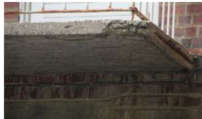
Rust on the Steel Bar
