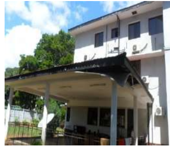
Ceiling board falling off
