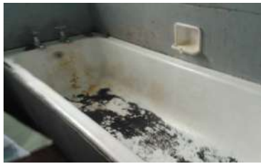
Bath tub not replaced
