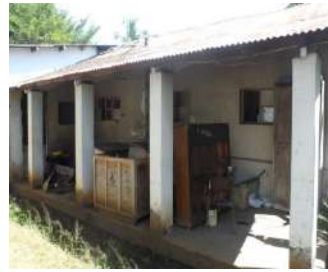
Unkempt servants quarter
