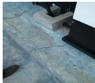
Cracks on the drainage
