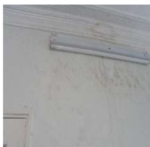
Leaking roof in the Conference Room at the top floor
