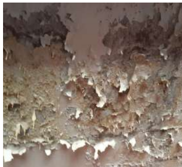
Damaged roof due to leakages on roof
