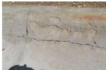
Cracked spoon drain
