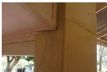
One of the cracks on the wall
