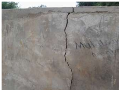
Crack on the wing wall of Chimowa dam
