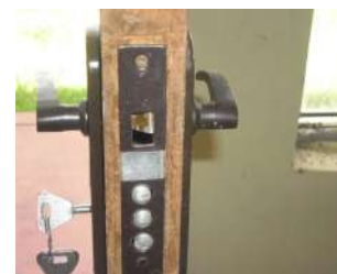
Defective Door Lock
