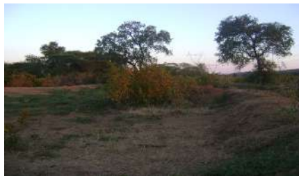
Shrubs in the spill way - Sikongo Dam
