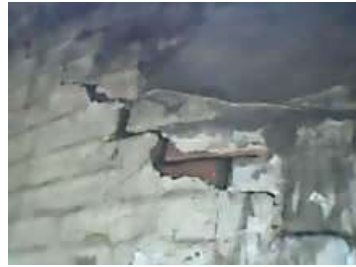
Crack on wall on one of the chalets
