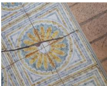
Crack on the dining room floor
