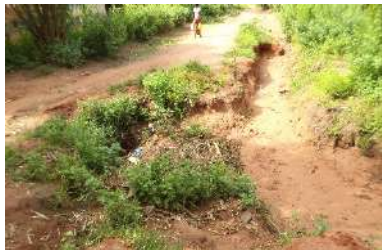
No drainages causing road erosion
