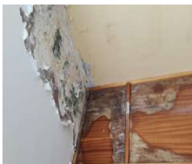
Damaged roof and furniture
