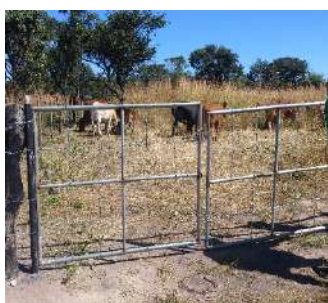
Gate secured with wires
