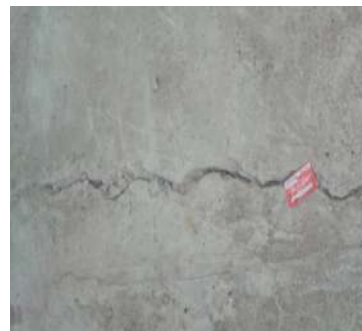
A Crack on Second Floor
