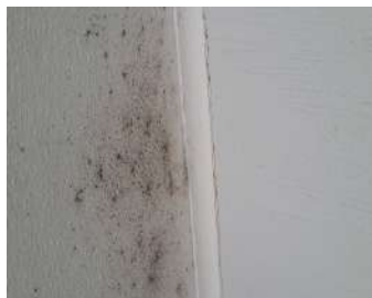
Leakage in the Kitchen
