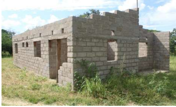
An incomplete Low Cost Staff House at Gable level at Ukwimi Basic School
