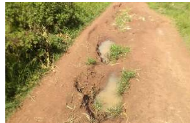
No drainages causing water ponding
