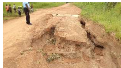
Blocked culvert and eroded road
