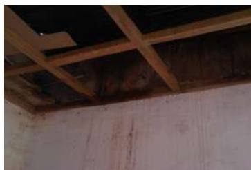
Leaking roof as evidenced by the stains on the walls
