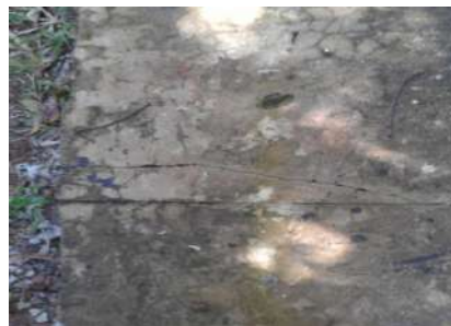
Cracks on the Apron
