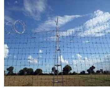
Incomplete razor wire on top of outer fence
