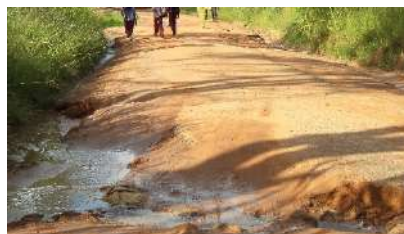
No drainages, water collecting in parts of road and road eroded
