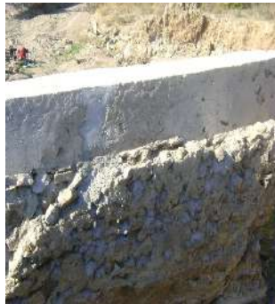
Mended crack on head wall
