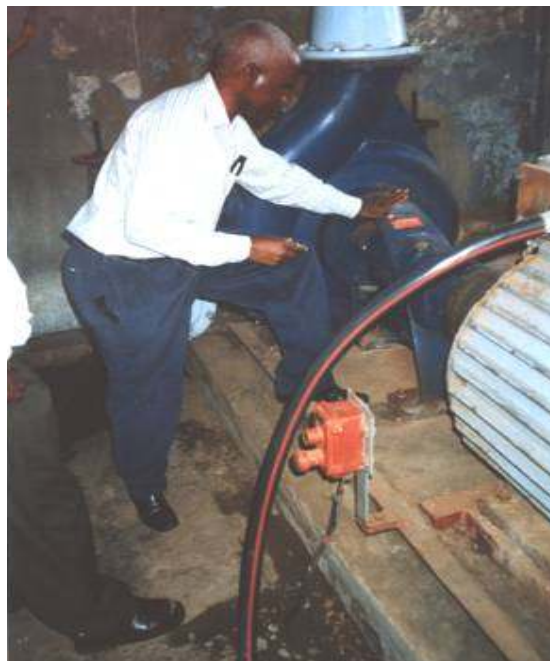
Non functional pumps mismatched to the motor
