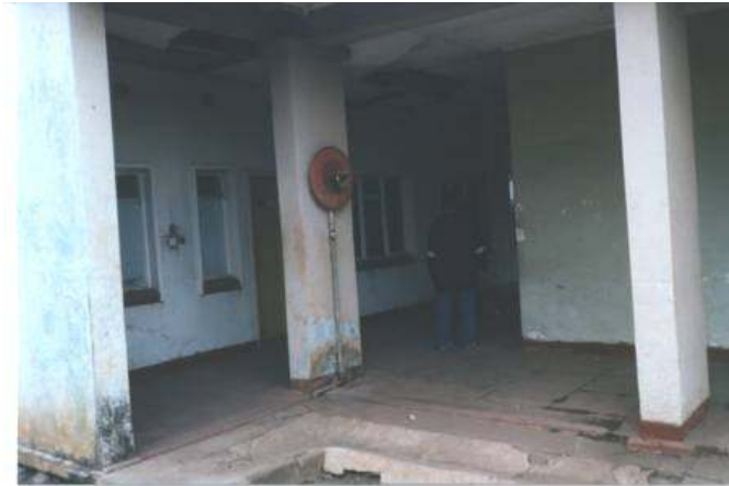
Part of the dilapidated building housing RTC and Government Stores
