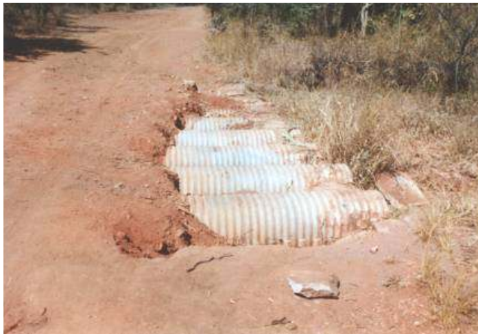
Eroded culvert along the 24KM formation (Zambian side).
