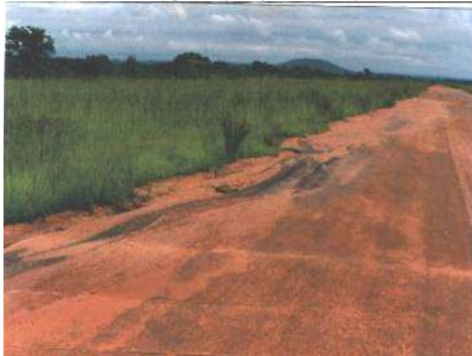
Deteriorated surface runway
