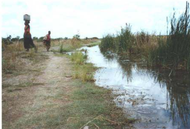
Leakages from the underground pipe Kalulu- Mukobeko
