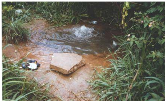
Water going to waste due to heavy leakages
