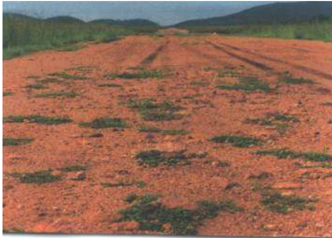
Washed away portion of the gravel main way.
