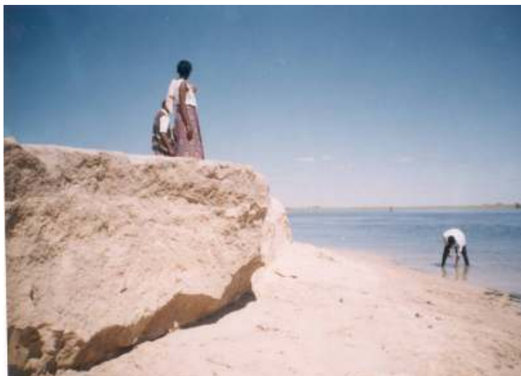
Portion of the washed away road
