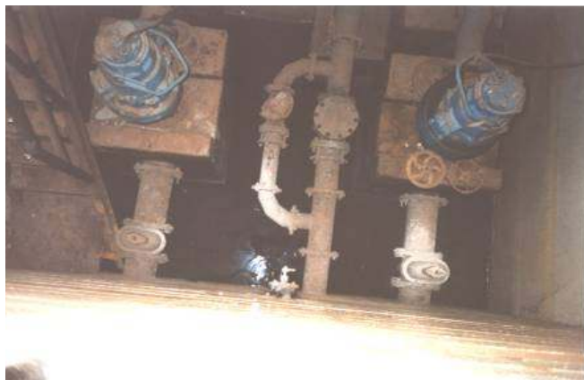
Two installed pumps but not functional
