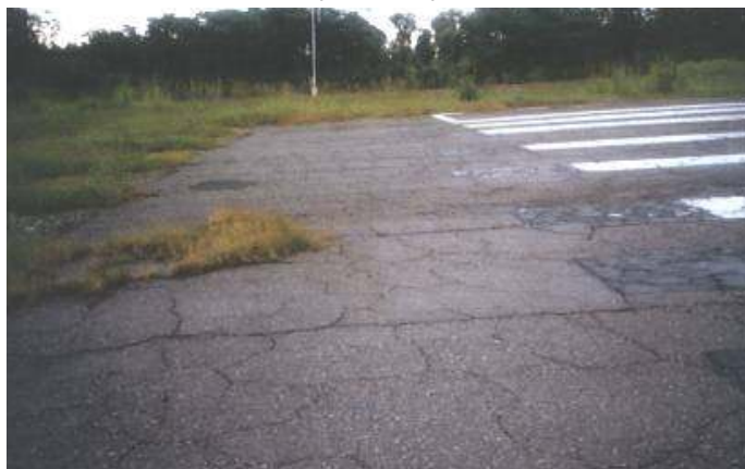
Poorly rehabilitated runway which led to additional works (slurry sealing)
