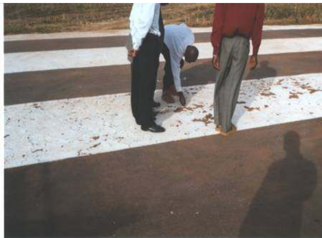
Paint peeling off due to chemical reaction at runway 18
