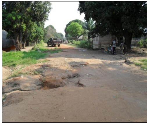
Wash out at 0.6 Km
