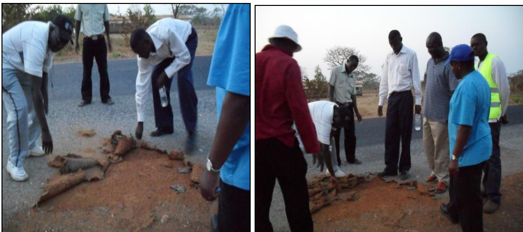
Peeling off of surface dressing of the road shoulders on all the reconstructed sections of the shoulders of the Chipata Lundazi road.
