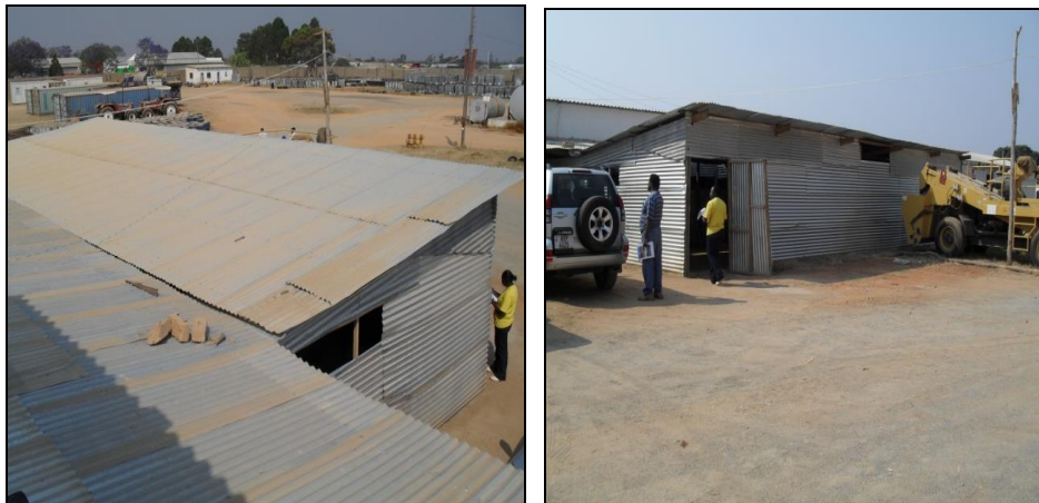
Sub standard structure established as extension of the Laboratory contrary to specifications
