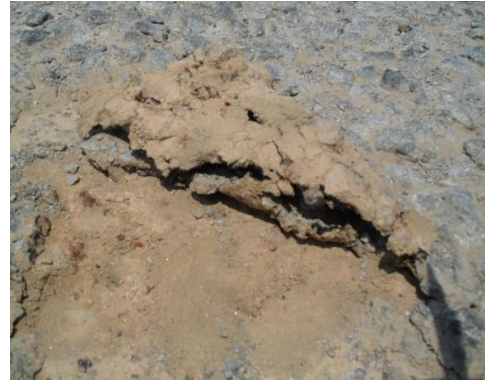
Lack of bond between the base and surface dressing on the shoulders
