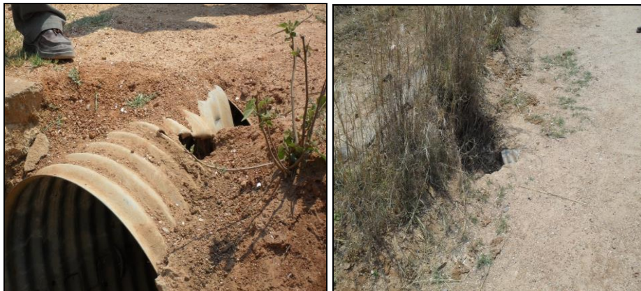
Damaged culvert at Km 62.7 and a blocked culvert
