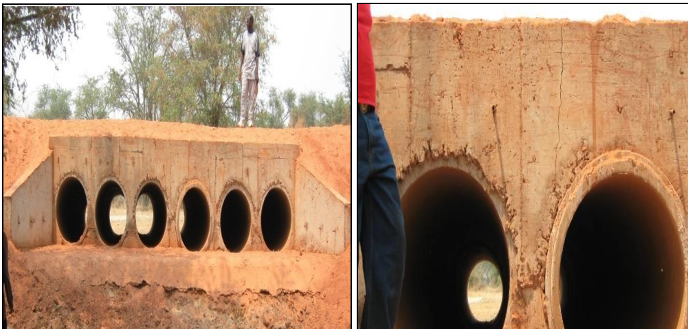
A six concrete culvert structure at KM 49.1 (LHS); A vertical crack in the middle (RHS)
