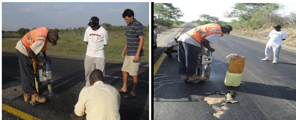
Collection of samples on re constructed sections of Maamba Batoka Road witnessed by contractor.
