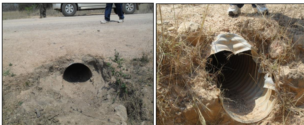
Culverts without head walls at km 41.7, and 58.2 kgalomo to Kabanga Mission road.
