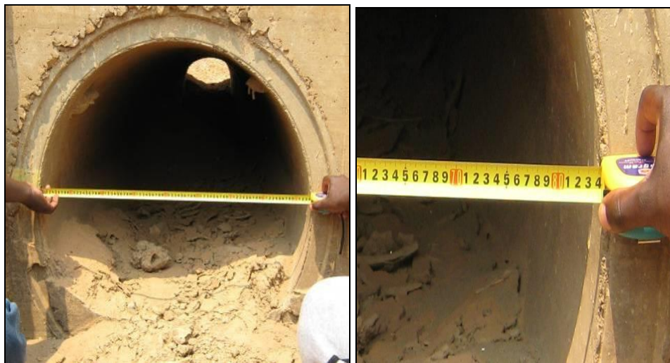
Culvert diameter measurement at KM 43.1(l) Internal diameter is 83cm instead of 90cm (r)
