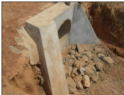
Poorly done culvert at Km 78.9 with no apron
