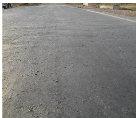
Signs of early bleeding on the surface KM 7+ 100
