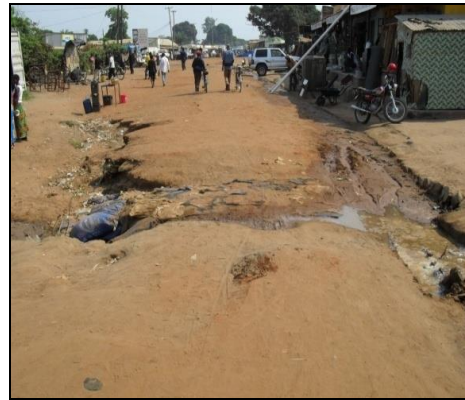
The carriageway eroded at 1.1km
