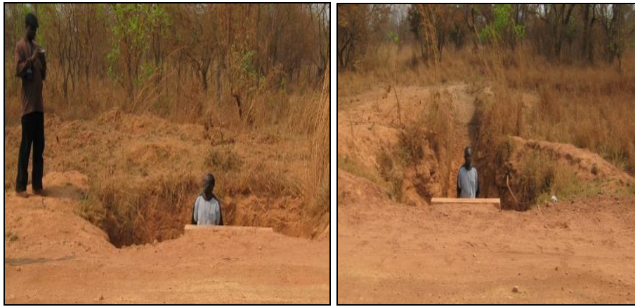
Culvert at KM 33.6: Inlet (LHS) and outlet having adverse slope (RHS)
