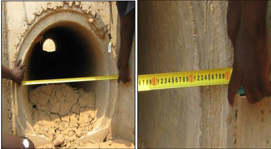
Culvert diameter measurement at KM 41.1(l) and Internal diameter at 83cm instead of 90 cm (r)
