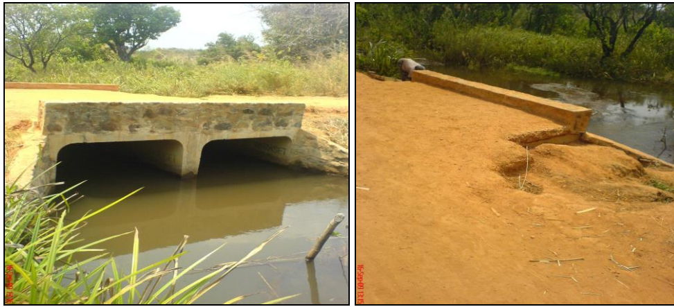
Completed Rosa Bridge (l) and Eroded Backfill on Newly Constructed Rosa Bridge (r)
