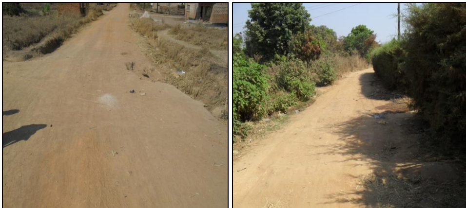
The wash out at 1.5 Km Part of the stretch with no formation at 2.6 Km to 3.0Km
