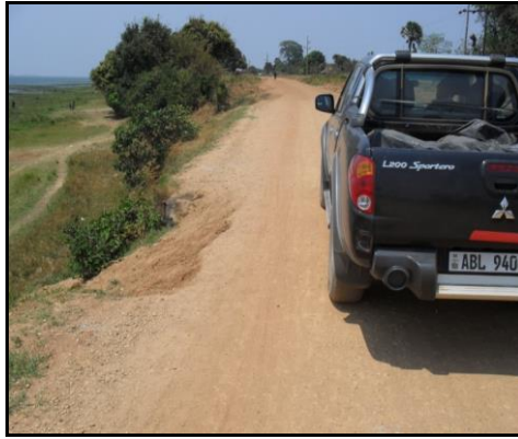
Erosion at Km 31.4 will affect the carriage way
