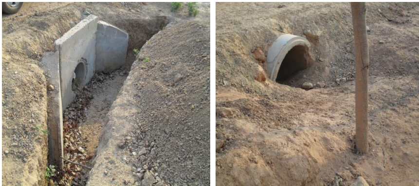
Culvert Headwall With Some Breakages Culvert Without Headwall
