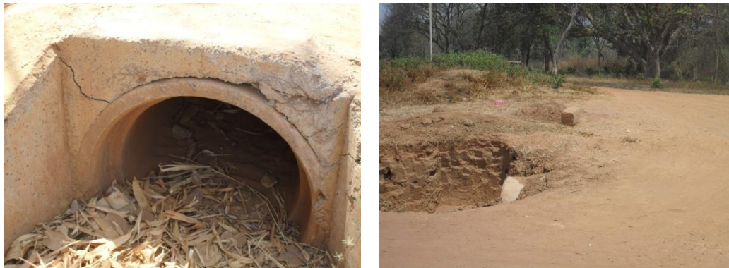
Cracked and Silted Culvert (l) & Without Headwall (r)
