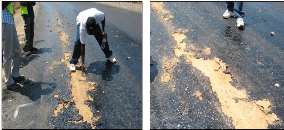
Officers effortlessly peeling off the surface dressing (l) and Failure on reconstructed sections between KM2.4 and KM50 (r)
