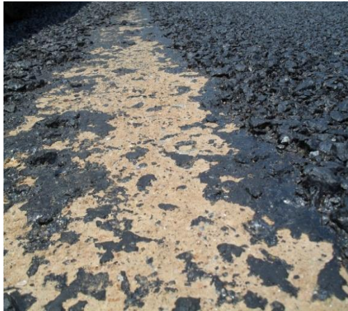
Peeling off of surface dressing layer from the base course
