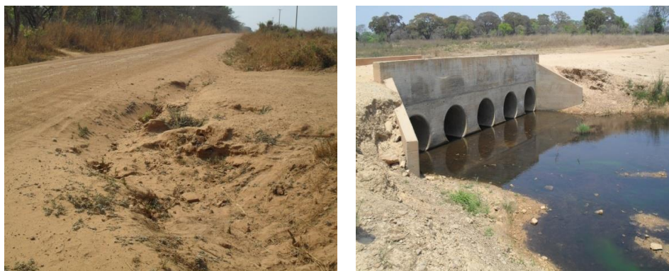
Eroded Road Side Drains and Culvert Wing Walls
