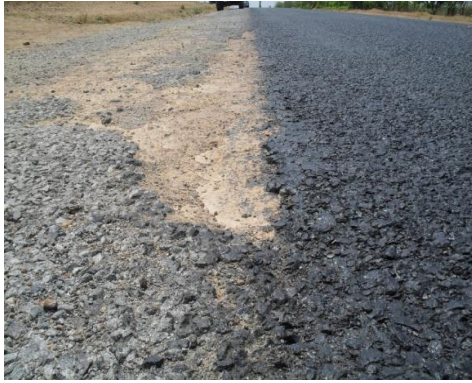
Peeling off of shoulder layer of surface
