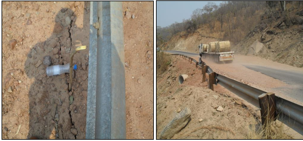
Cracks and a culvert without an inlet on the temporal works
