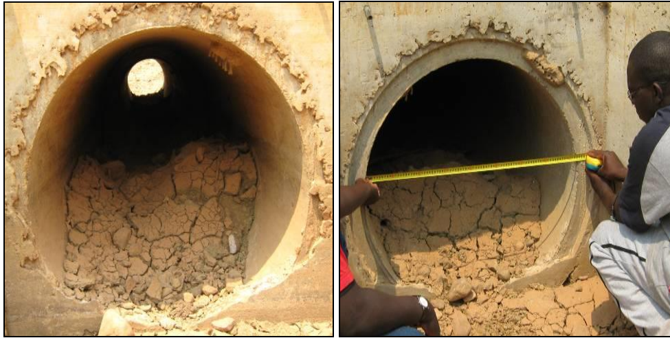
Unattended partially blocked culverts at KM 41.1 and 42.5
