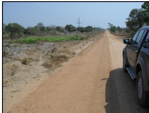
Mitre drain not discharging water at Km72.7
