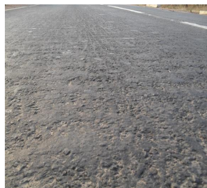
Corrugations on the surface KM7.1
