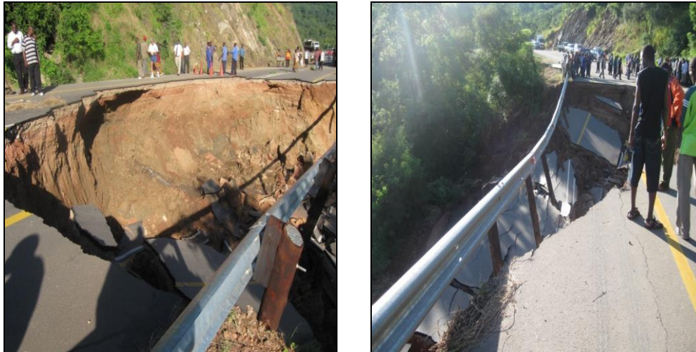
Failure of the road at 100 + 900 KM from Lusaka
