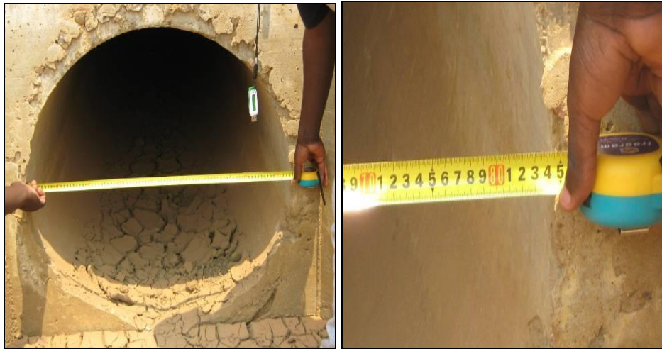
Culvert diameter measurement at KM 53.9 (l) Internal diameter is 84cm instead of 90 cm (r)
