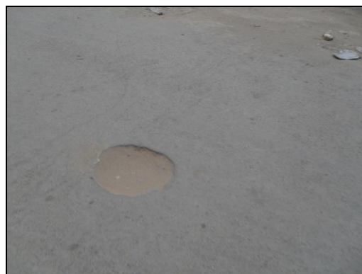
Pothole on the car park in Solwezi
