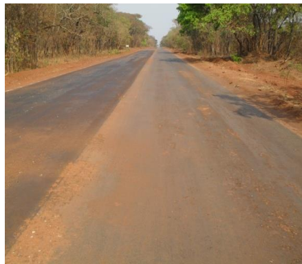
Damaged primed road surface
