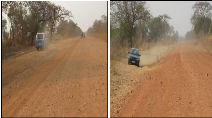
Vehicles preferring roadside track due to poor riding quality of the roadway (KM 6.7)
