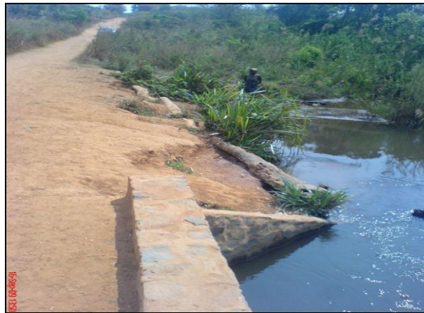
Eroded Approaches on Newly Constructed Rosa Bridge
