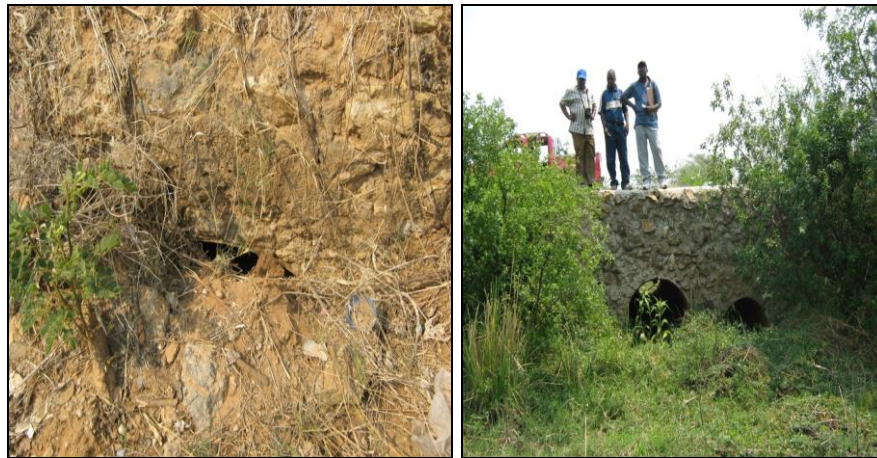
Fully silted culvert at KM 53 (l) and Culvert at KM 12.1 partially silted with overgrown vegetation (r)
