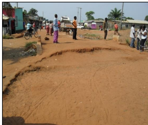
No road formation at 1.3 Km could not be used because of a wash out
