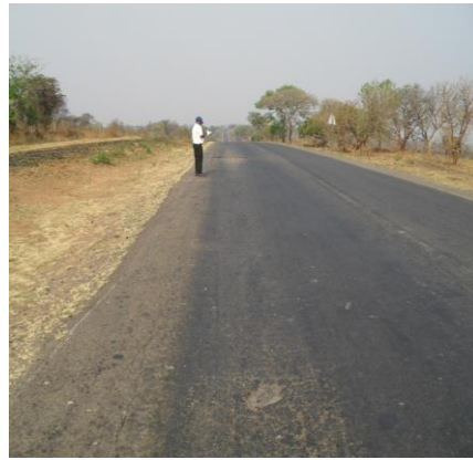
Cracks and potholes near Chikankata turn off
