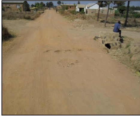
Poorly constructed drift at 1.6 Km (l)
