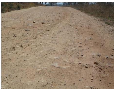
Poor/Rough Road Surface on State Lodge at chainage 0+100 to 0+400
