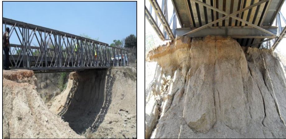
Temporal bridge not included in permanent works (l) and Wide cracks including signs of erosion (r)
