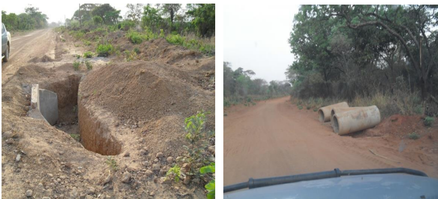
Culvert without inflow/outflow drains Culvert pipes awaiting installations
