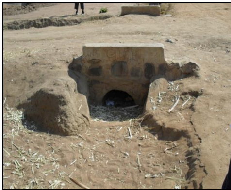
Poorly constructed culvert at 1.6 km With base a concrete washed out already silted
