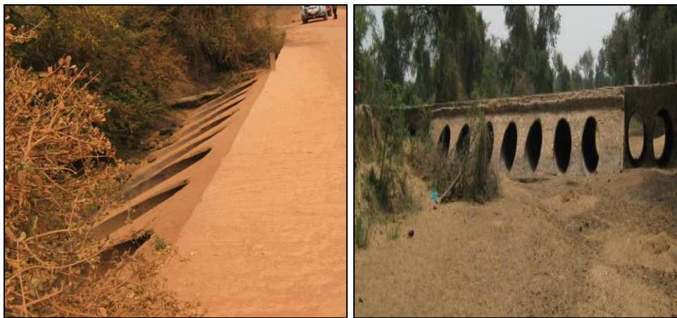
Unattended vented drift inlets with vegetation partially blocking vent openings at KM 35.8 and 48.5. No edge marker posts for traffic safety during overflow situation
