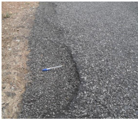
Edges not repaired surface dressing properly prior to
