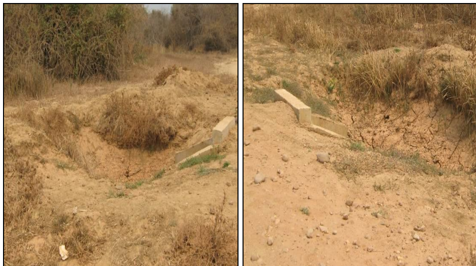
Culvert at KM 41.1: Drop inlet (LHS) and outlet with no outfall ditch (RHS)
