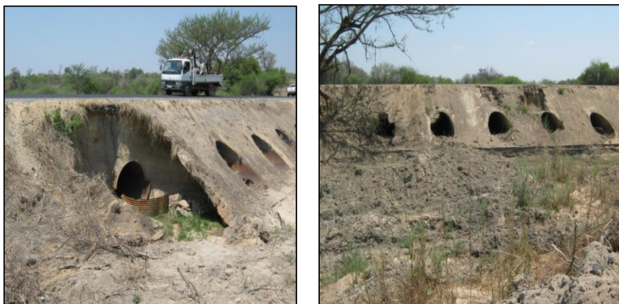
Erosion on newly re-constructed pavement(l) and Lack of protection works on new road (r)
