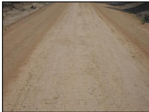
Cracks on the carriage way. Starting from Km71.9 to Km80.0
