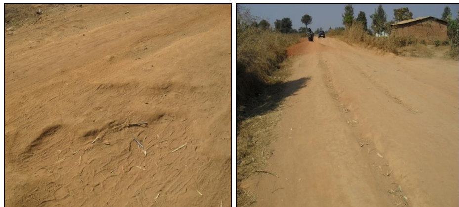
The pothole at 0.9 Km Truck mark on the road at 1.7 Km
