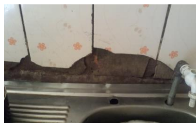
Cracked wall tiles
