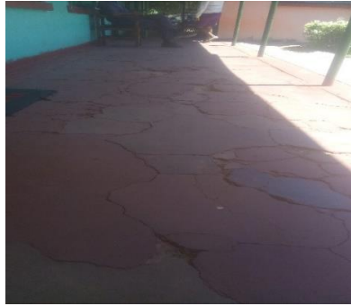
Cracked corridor floors
