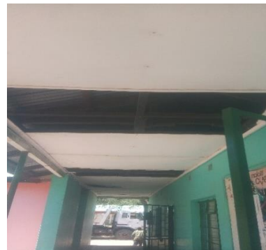
Ceiling Board at Council Offices
