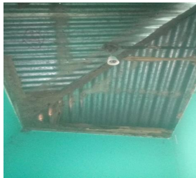
Ceiling Board eaten by termites
