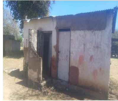
Dilapidated outside toilets
