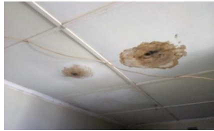
leaking roof at the reception entrance
