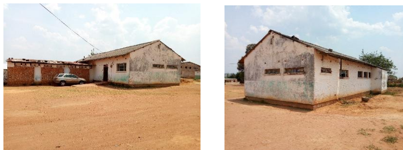
Dilapidated building - Bantungwa Tarven
