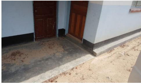
No spoon drain was done
