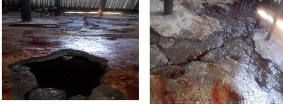
Abattoir floor with potholes and cracks
