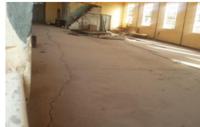
Cracks on the floor
