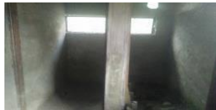
Toilets without toilet pans fitted in the Gents
