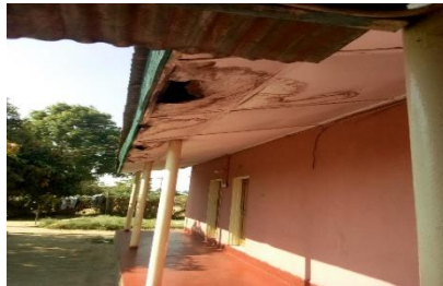
Damaged ceiling board in corridor
