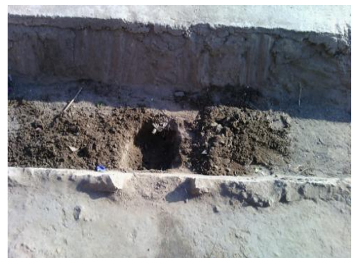
Drainage without a lined base along Chipata 2 road (Lot 8 B11)
