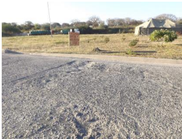
Worn out driving surface at Kazungula Weighbridge
