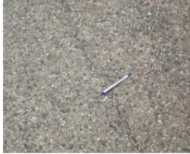
Reflective Cracking on the road surface.
