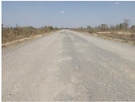
Worn out crushed stone base not protected with quarry dust from weather elements and traffic
