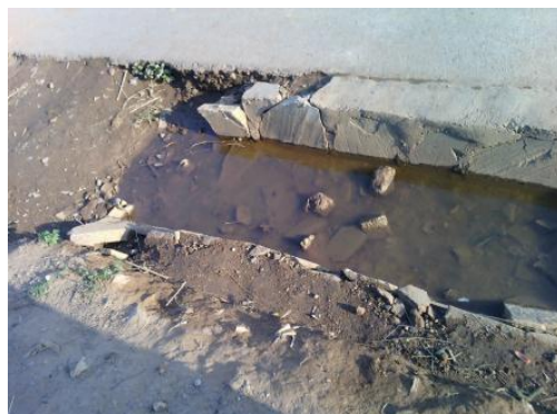
Lack of access for continuous flow of water along Chipata 2 road (Lot 8 B11)
