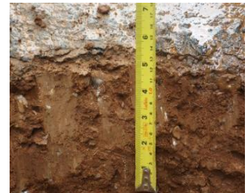
A trial pit on Nkholoma Stadium Road with a stabilised base thickness of 110mm.
