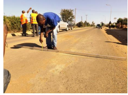
Rutting of 12mm under a 3m straight Edge
