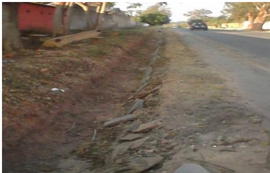
Incomplete Drainage Structure in Chudleigh due to Inadequate BOQ Materials (Lot 8 B10)
