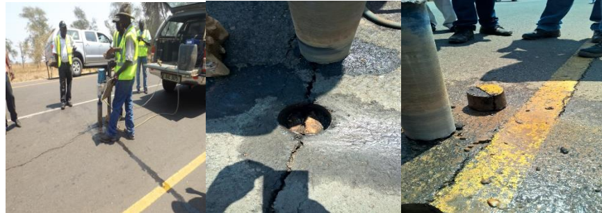
A core taken on the crack reviewed that the cracks propagated all the way to the base
