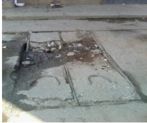
Installed concrete slabs breaking up on drainages along Chozi Road installed concrete slabs wearing out with Y10 bars showing (Lot 8 A5)
