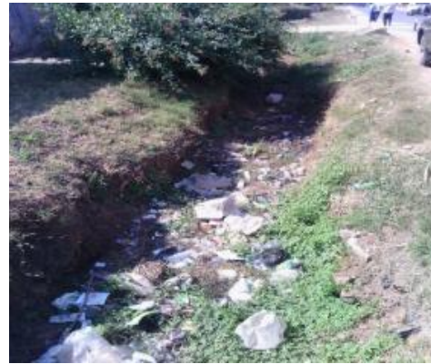
A section of the road measuring thirty (30) metres had no stone pitch on Ngwerere road in Chelson Square pitch (Lot 7 A4)
