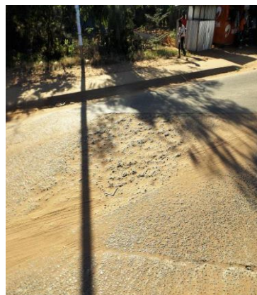
Area prone to water logging with poor design leading to base failure
