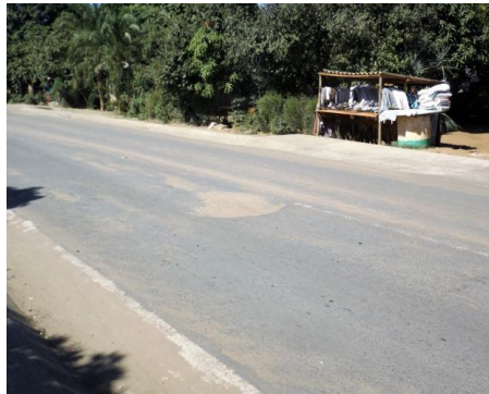
Area prone to water logging with poor design leading to base failure
