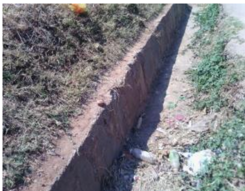
Incomplete Drainage structure (Lot 7 A4) Structure stone pitched on one side(Lot 7 A4)
