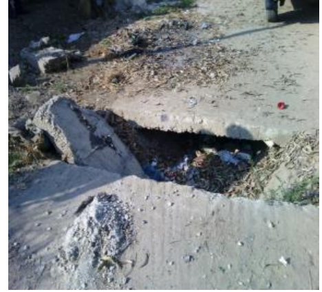
Parts of concrete slabs installed along Chozi Road had broken (Lot 8 A5)
