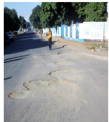
Area prone to water logging with poor design leading to base failure
