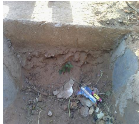
Drainage with dead end as there was no provision of access to private property (Lot 8 B11)
