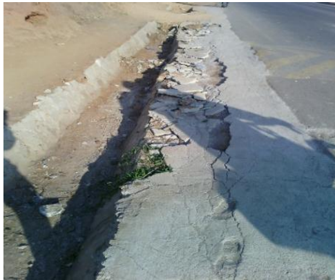
Constructed shoulders and walk way without conforce wire breaking up along Chipata 1 road (Lot 8 B11)
