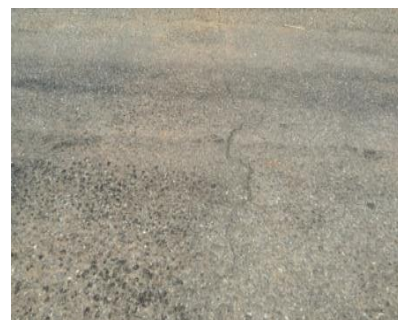
Cracks on the newly constructed road
