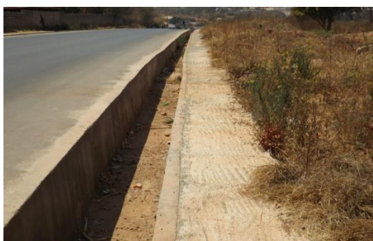
The walkway with bad aesthetics and no expansion joints
