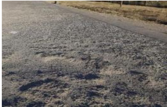
Poorly constructed carriageway reinforced with conforce wire
