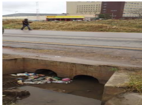
The NASDEC Road had a drainage system that did not have an outlet for the storm water leading to ponding at the entrance to the Showground
