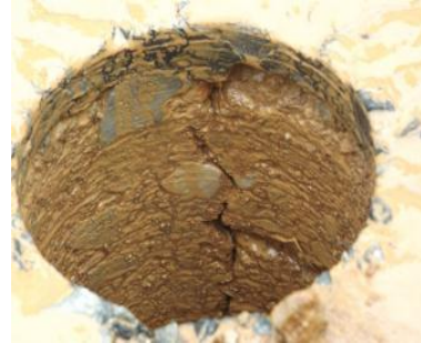
Evidence of reflective cracking going through the base.
