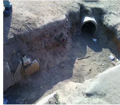
Incomplete works with stones falling off at Chipata 1 road (Lot 8 B11)
