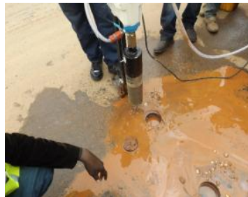
A core on Nkholoma Stadium road retrieved without any Base Material
