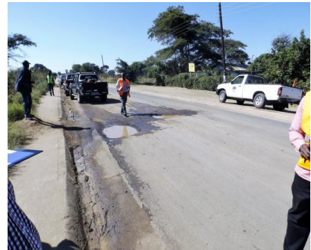
Poor drainage design
