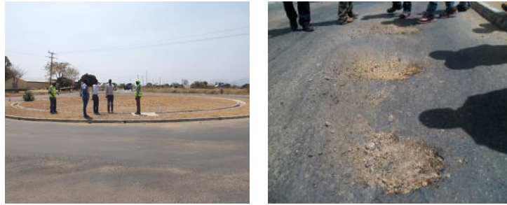
Potholes and rutting at the roundabout has not yet been repaired.
