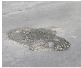
Pothole on Mukuba Road
