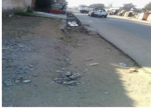
Incomplete/abandoned drainage works along Mutendere road (Lot 7 A3)
