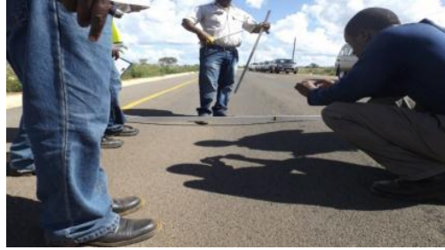
Surface Irregularity at 34mm on the average cross section on road No. 1 in MFEZ area
