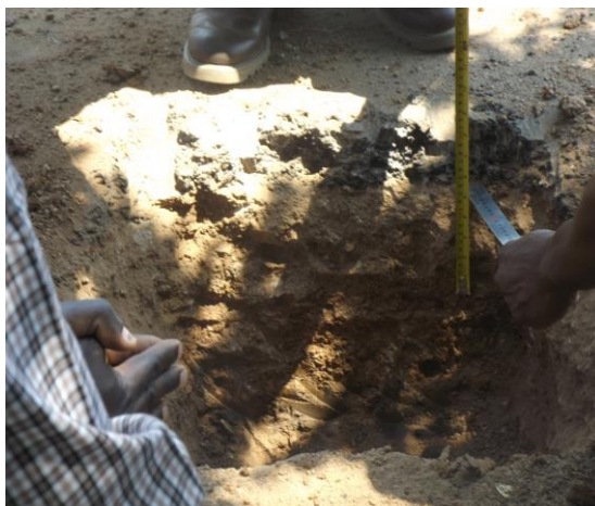
Trial Pit along the road from Mfuwe to the Gate to South
