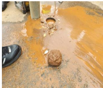
A core on Nkholoma Stadium road retrieved with a stabilised base thickness of 50mm contrary to the required 150mm.
