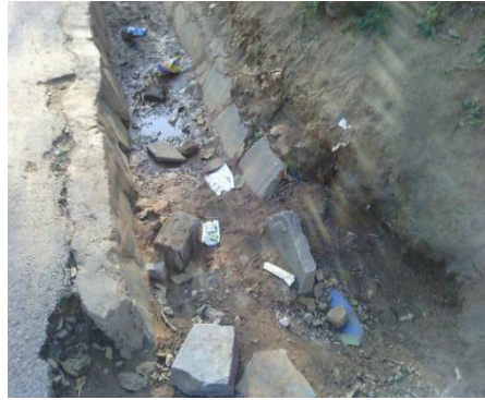
Drainage structure on Chipata 1 road without a concrete lined base (Lot 8 B11)
