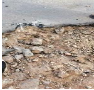
Existing mine waste rock road base used as opposed to crushed stone base
