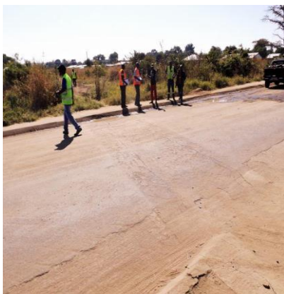
The concrete on the Dip was poorly designed affecting smaller vehicles, it was repaired unconventionally
