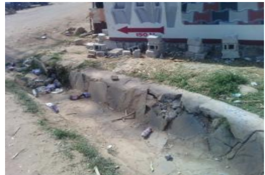
Broken Drainage structure at the Mutumbi Curve (Lot 7 A3)
