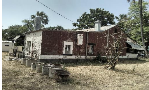
Dilapidated vacant house
