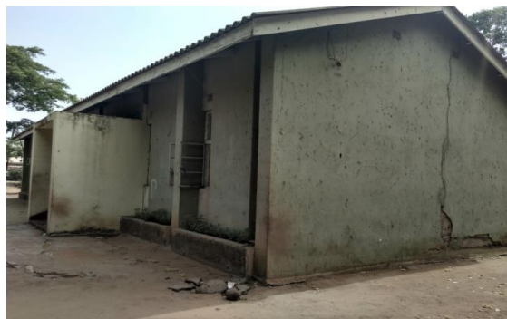
Dilapidated building in Dambwa North
