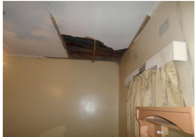
falling ceiling in one of the motel rooms
